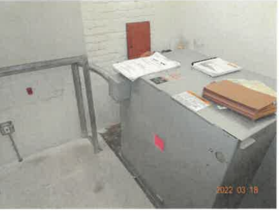
36. View of the elevator pump unit.
