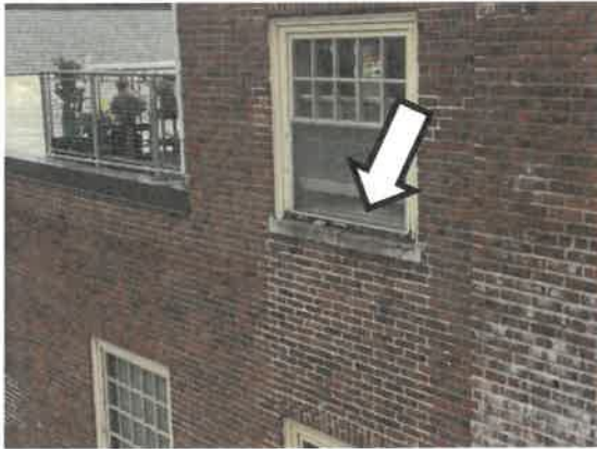
Photo 7 – View of deteriorated wood at an isolated window sill.
