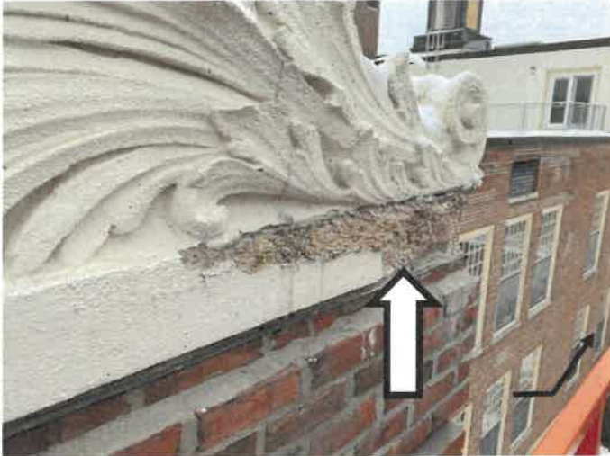
Photo 9: View of a spall in the bottom of a decorative cast stone coping at the rear east elevation where Gale observed the removal of loose delaminated cast stone. Refer to Photo 10 for side elevation view of the cast stone spall.
