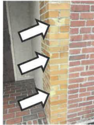
Photo 10 – Spalled yellow glazed brick masonry.
