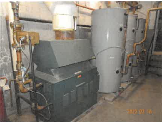
39. View of the domestic hot water (DHW) system.
