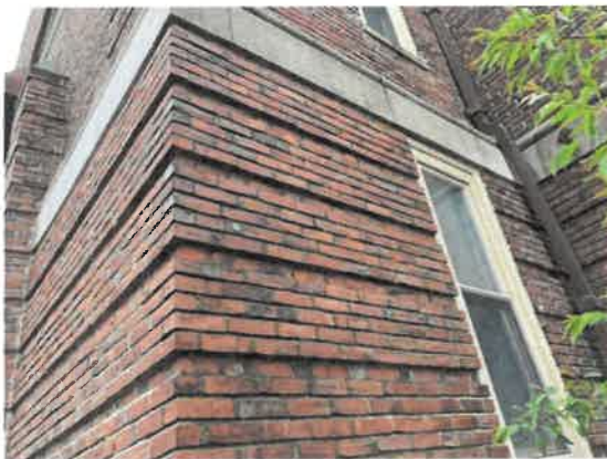
Photo 3 – View of deteriorated mortar.
