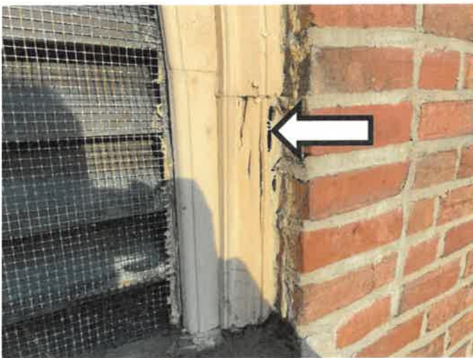
Photo 7: View of split wood frame around the louver at the rear east gable roof. Gale observed deteriorated wood framing at isolated locations around the louver penetrations.
