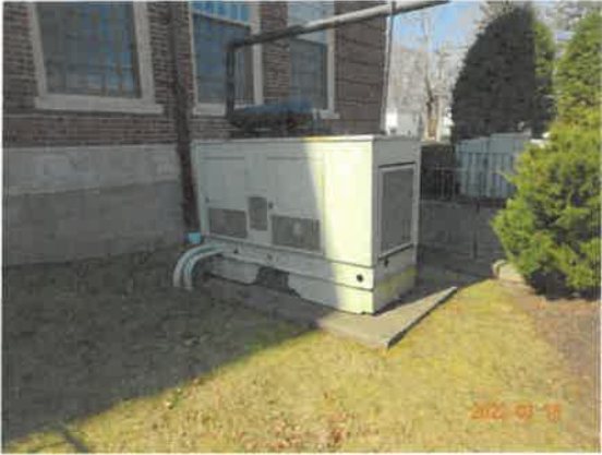
32. View of the original emergency generator.
