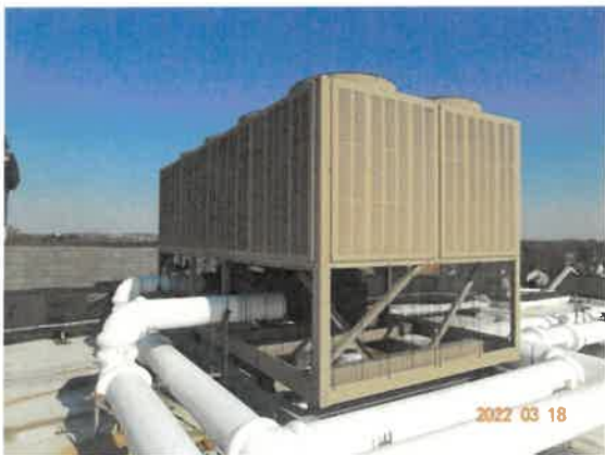
41. View of the rooftop chiller.
