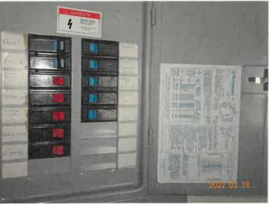
30. Typical view of the unit circuit breaker panels.
