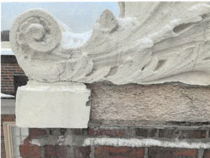
Photo 3: View of multiple cracks along the decorative cast stone coping, where water infiltration can occur.
