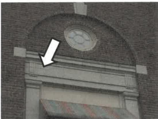
Photo 5 – View of cracked precast stone.
