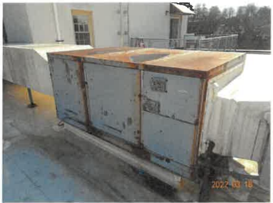
42. View of the rooftop HV units that provide common area space heating.
