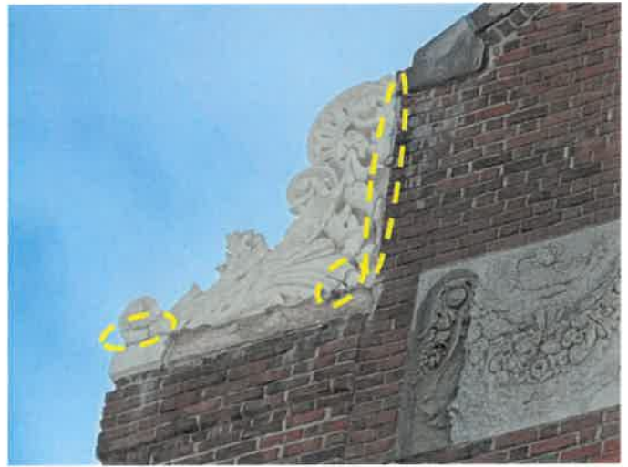
Photo 8: View of temporary crack repair at the rear east decorative cast stone coping. The temporary repair included the application of sealant along the cracks to limit water infiltration.
