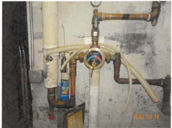
40. View of the DHW mixing valve.
