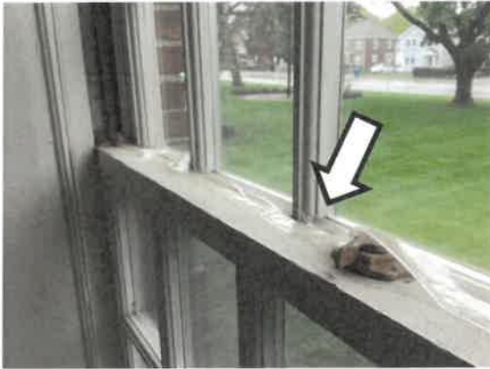
Photo 3 – View of tape installed between the sashes at an isolated window unit.
