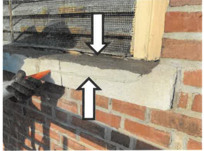
Photo 6: View of a temporary sealant repair of a crack in the stone beneath the louver penetration. Gale observed a gap between the vent and the stone sill, which is a path for water infiltration. The gap between the vent and the stone sill was sealed with sealant to limit water infiltration.
