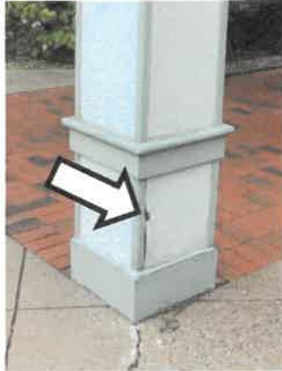
Photo 1 – View of damaged wood trim at entrance canopy.
