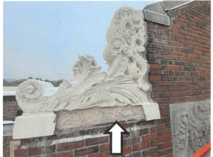
Photo 2: View of the front east decorative cast stone coping, where the bottom of the cast stone fell prior to Gale's arrival.
