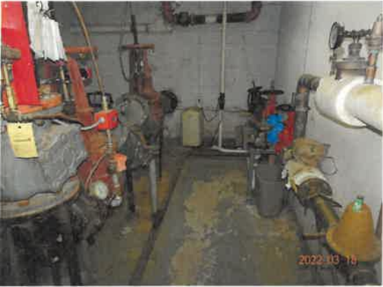
33. View of the incoming water and sprinkler lines. Both have double check backflow preventers installed.
