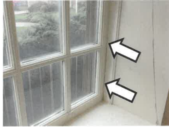
Photo 6 – View of window sash painted shut.
