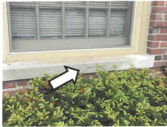
Photo 4 – View of a cracked precast concrete sill.
