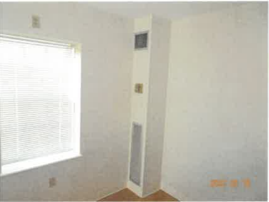
29. Typical view of a vertical WHALEN unit that provides heat and air conditioning to the units.
