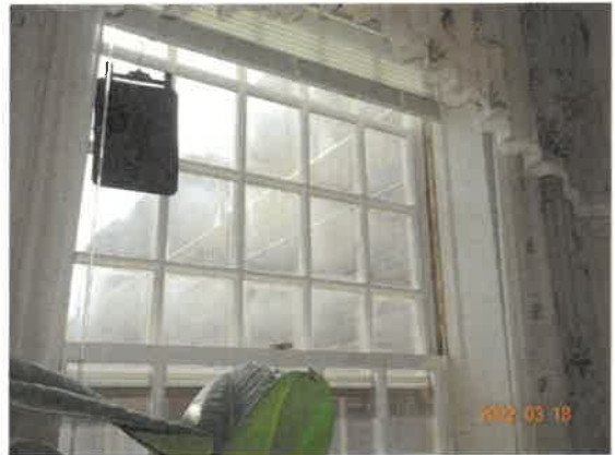
10. Window frames include a mix of decorative wood and aluminum. Some fogged lites noted.
