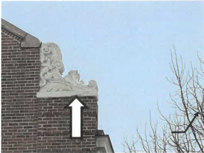
Photo 5: View of a spall at the base of the decorative cast stone coping at the rear west elevation.
