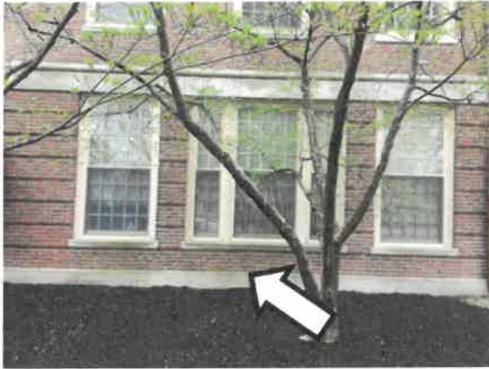
Photo 7 – View of vegetative staining below window units.
