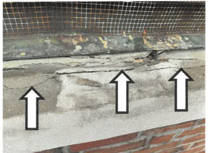
Photo 8: Closer view of the cracks and delaminated stone along the sill at the rear east gable roof. Gale observed a gap between the bottom of the vent and the stone sill, which is a location for water infiltration.
