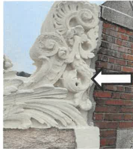
Photo 4: View of a full height crack in the decorative cast stone coping at the front east elevation. Colonial applied sealant to the cracks to limit water infiltration that were identified by Gale.
