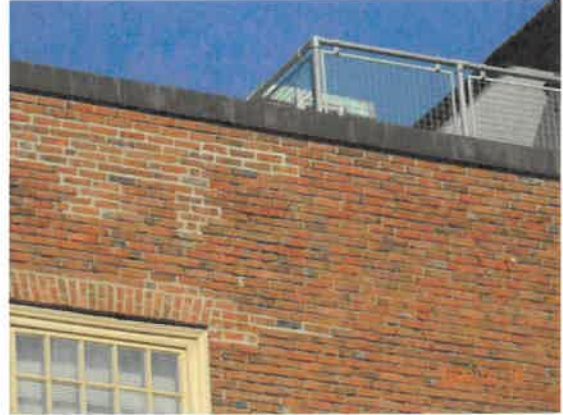
8. Some areas of the brickwork have been repointed. Some areas are in need of repointing.
