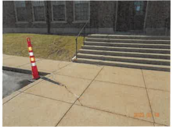
4. View of the concrete walkways. Some areas of the concrete exhibits cracks and the curbs exhibit some damage.
