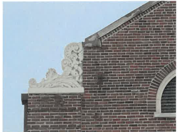
Photo 6: View of a temporary repair of a full height crack in a decorative cast stone coping at the front west elevation. The temporary repair consisted of the application of sealant along the crack.
