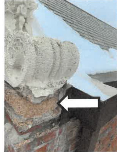
Photo 10: Side elevation view of the spall where Gale observed loose delaminated cast stone. The gable roof gutter was observed to be behind the decorative cast stone coping.
