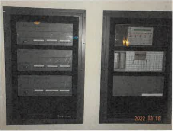
34. View of the central fire alarm panel. The panel was recently replaced.
