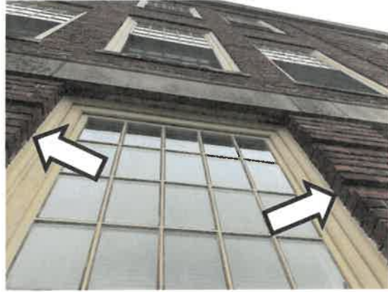
Photo 8 – View of failed perimeter sealant at an isolated window unit.
