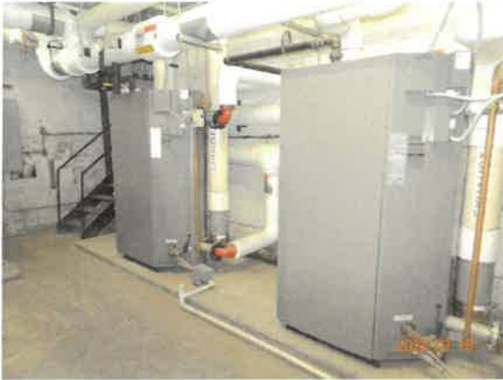
37. View of the main heating boilers. All replaced.
