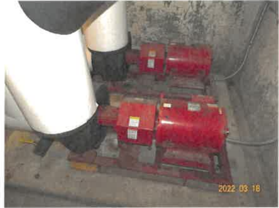
38. View of the heating and chilled water circulators. Good condition.
