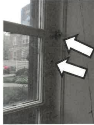
Photo 4 – View of the retrofitted limit stop installed at a window unit in the former pre-school.
