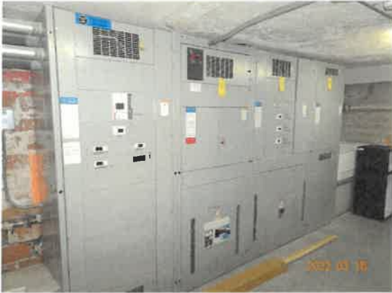
31. View of the main electrical panel.
