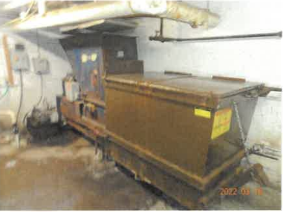
35. View of the trash compactor.
