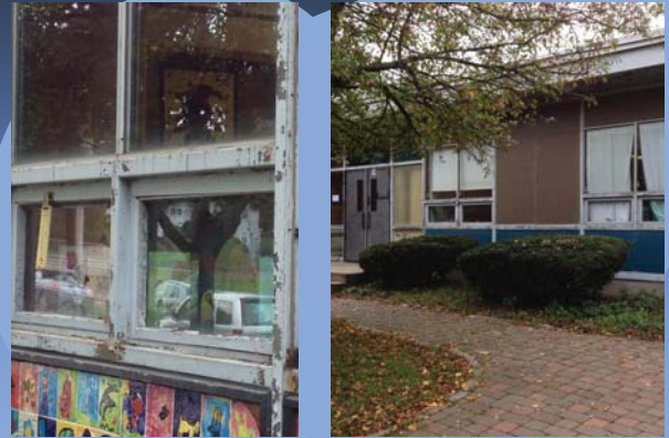
Cabot – Window and Door Deterioration
