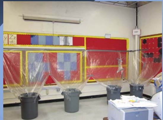
Angier – Water Infiltration
