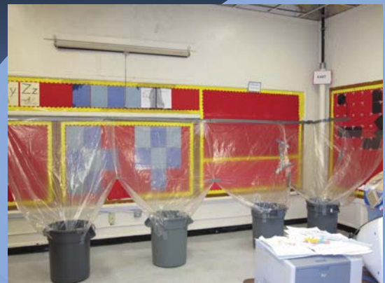
Angier – Water Infiltration
