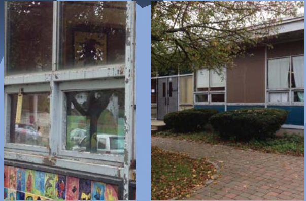
Cabot – Window and Door Deterioration
