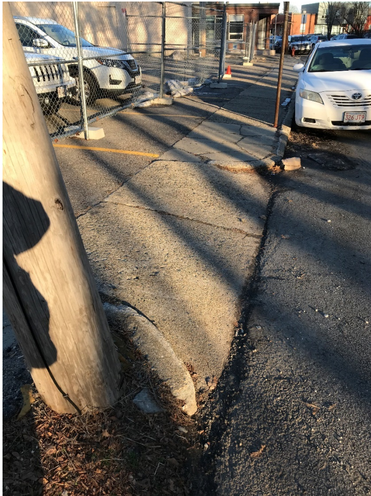
This driveway apron needs to be closed & remodeled
