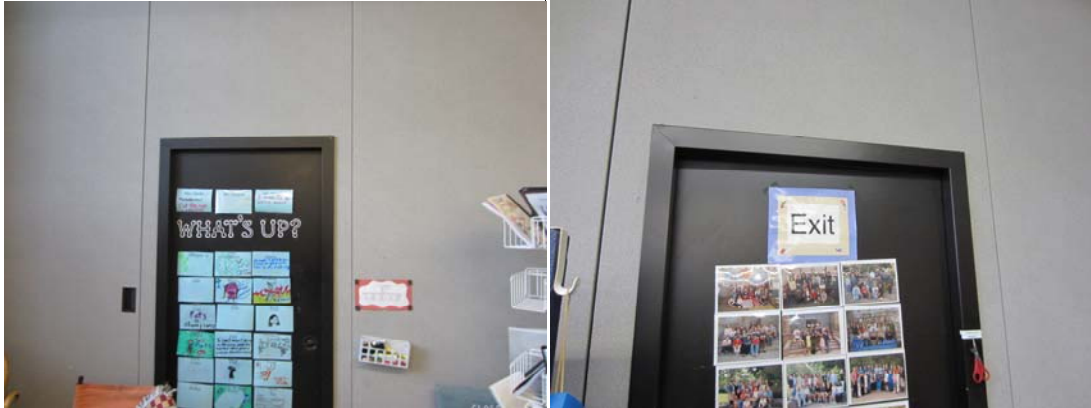
Zervas - Exit signage required
