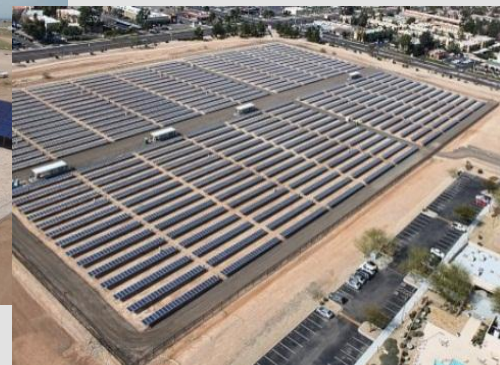
2 MW, Arizona State University
