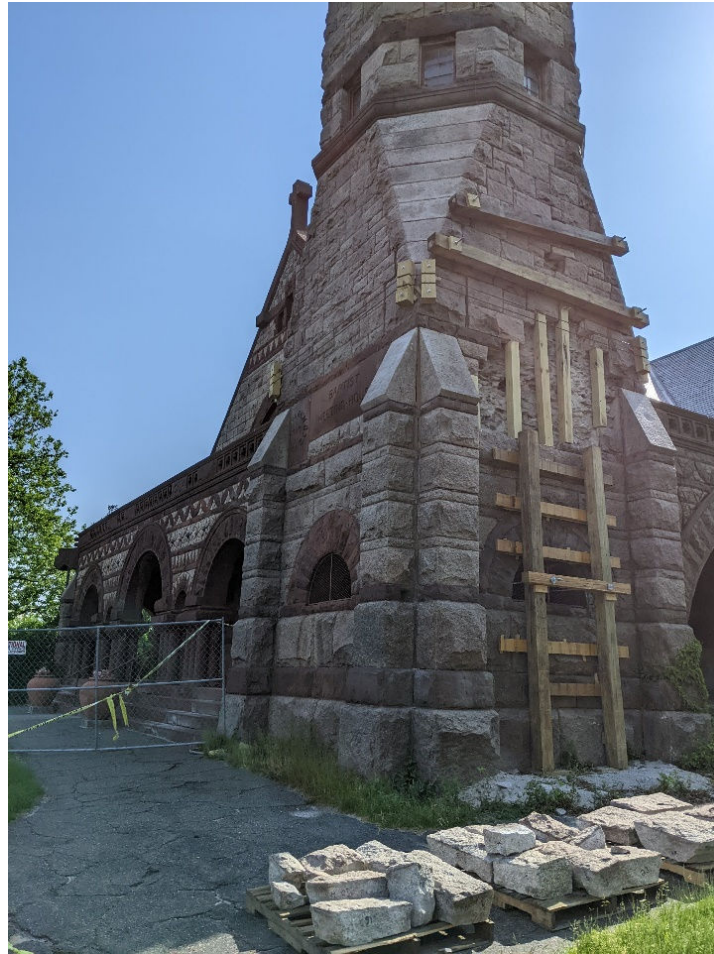
Dunnage and emergency brace. Marked and inventoried stones preserved on pallets for reinstallation.
