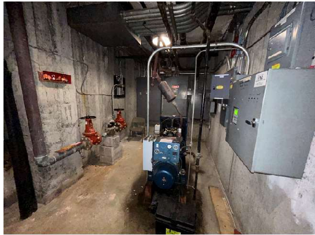
Generator Room, Ground floor (10)
