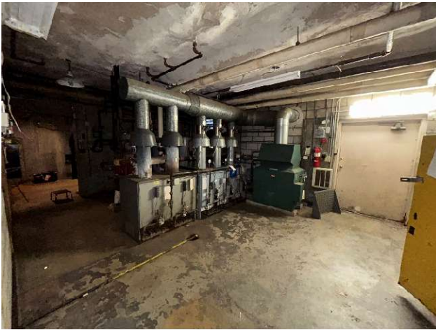
Boiler Room Ground floor (9)
