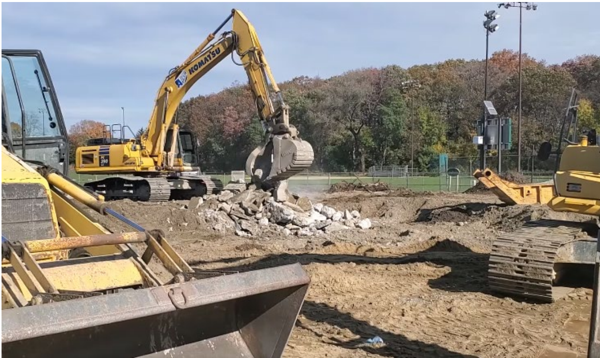
The contractor has completed the demolition of the pool shell, deck, and other site elements.
