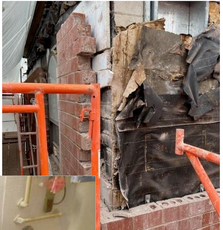
Asbestos and Failing Structure
