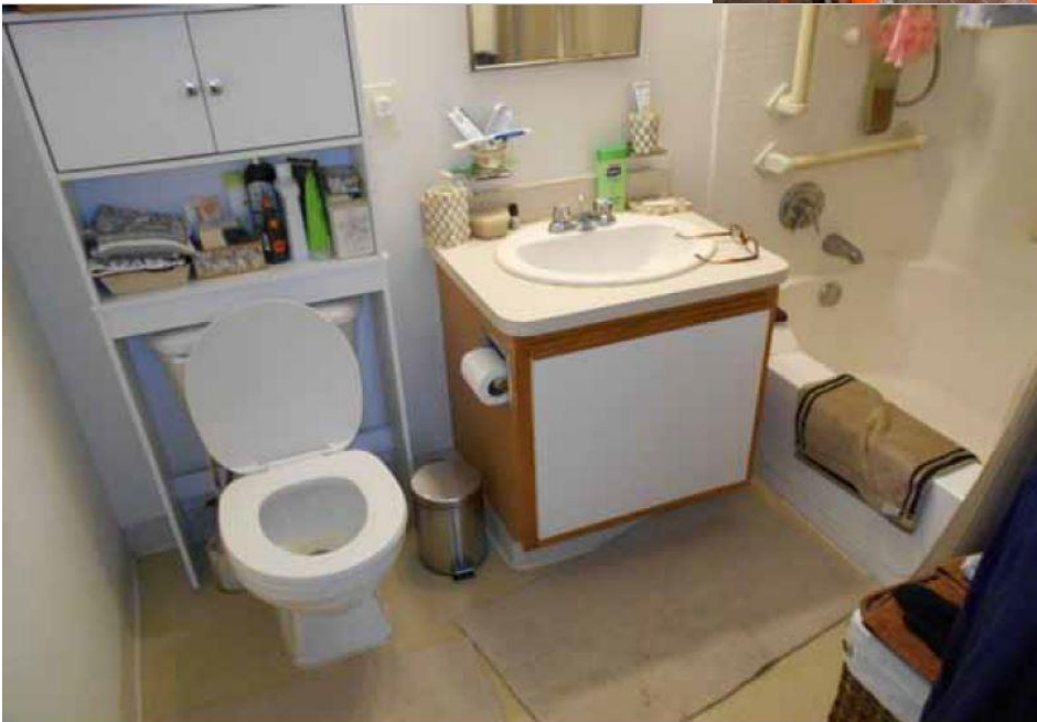
Non-compliant bathrooms with tubs
