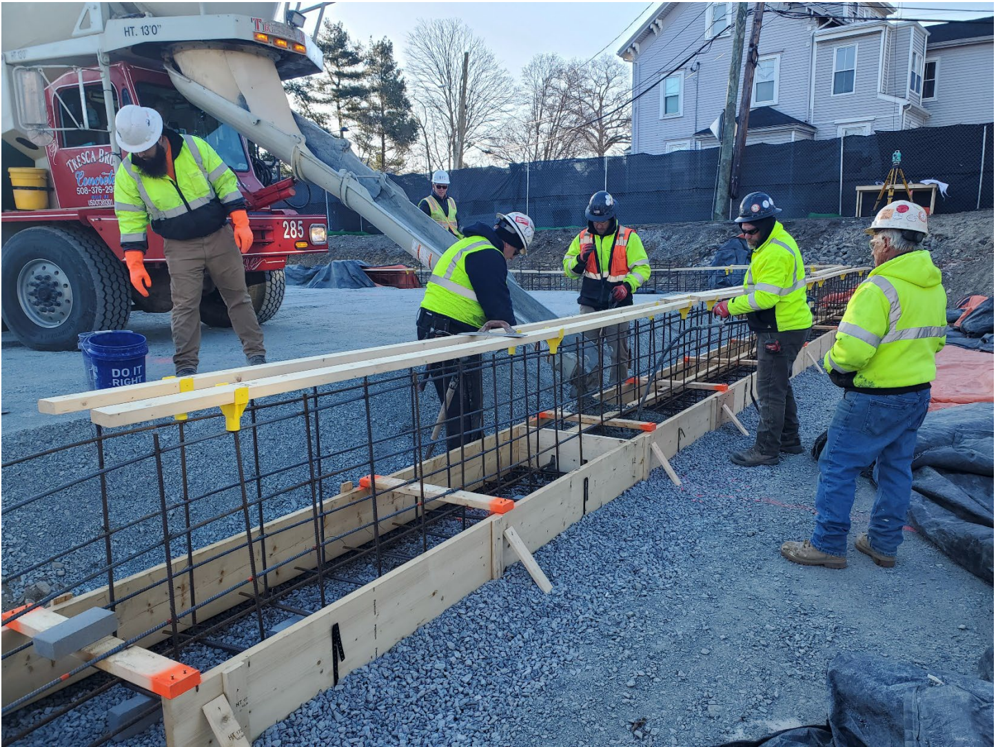
A few weeks back the team from J&J Contracting poured the first concrete to establish our foundation for the new Cooper Center.
