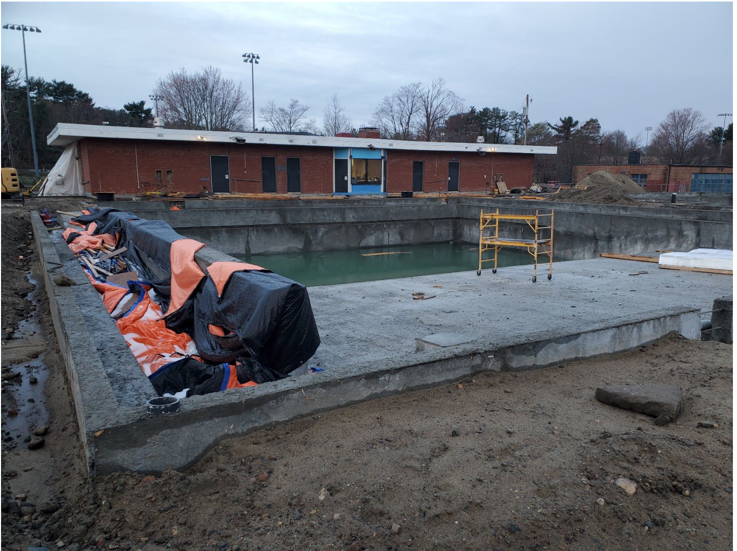
The two new pools are fully poured, and the new pool gutters are being installed. On the left you can see the ramp that will allow people of all abilities to enjoy the competition and lap pool. The splash pads will be located to the right of this image.
