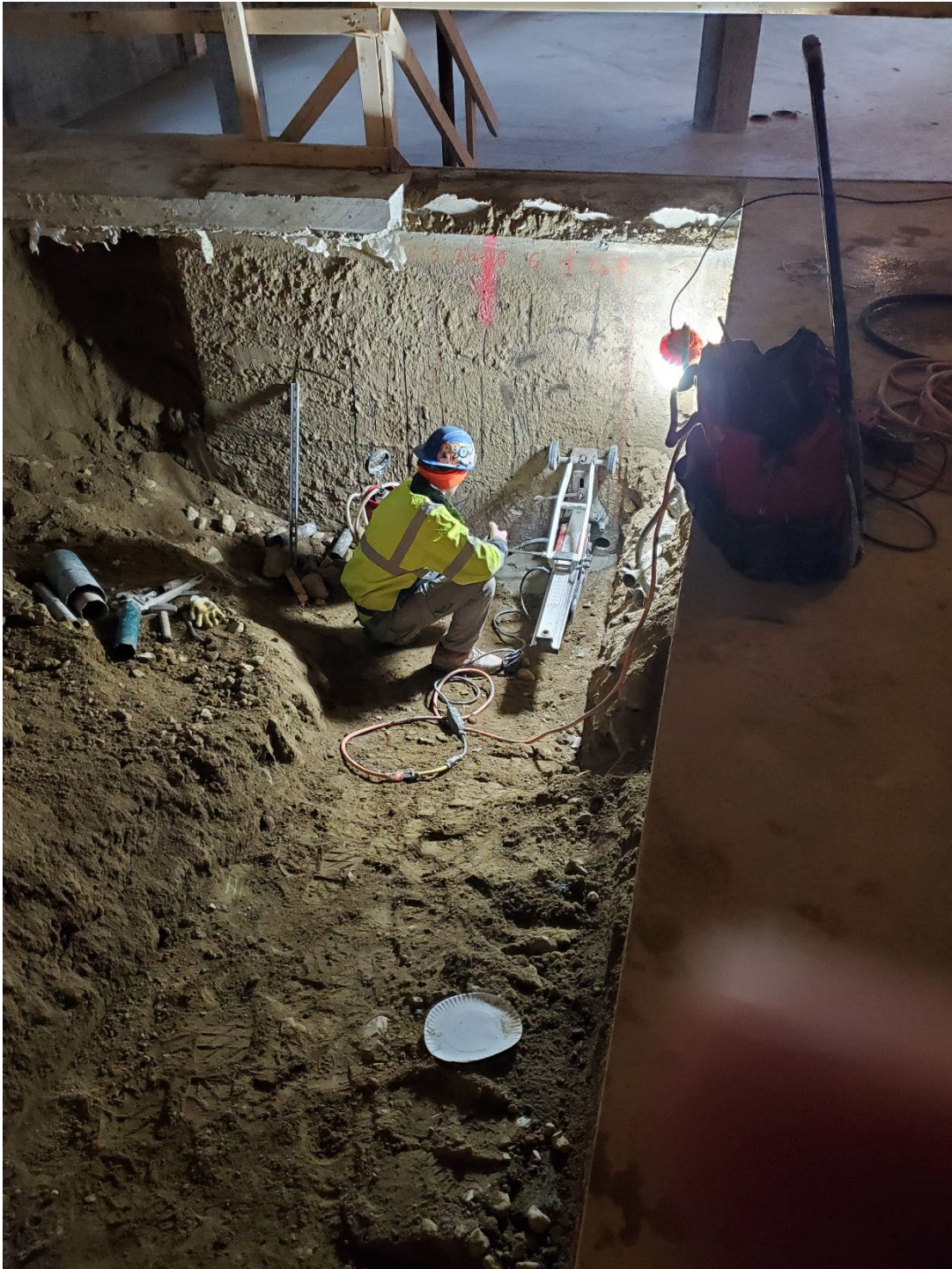
In the above picture, one of our electricians is coring holes to make way for the new electrical conduits.
