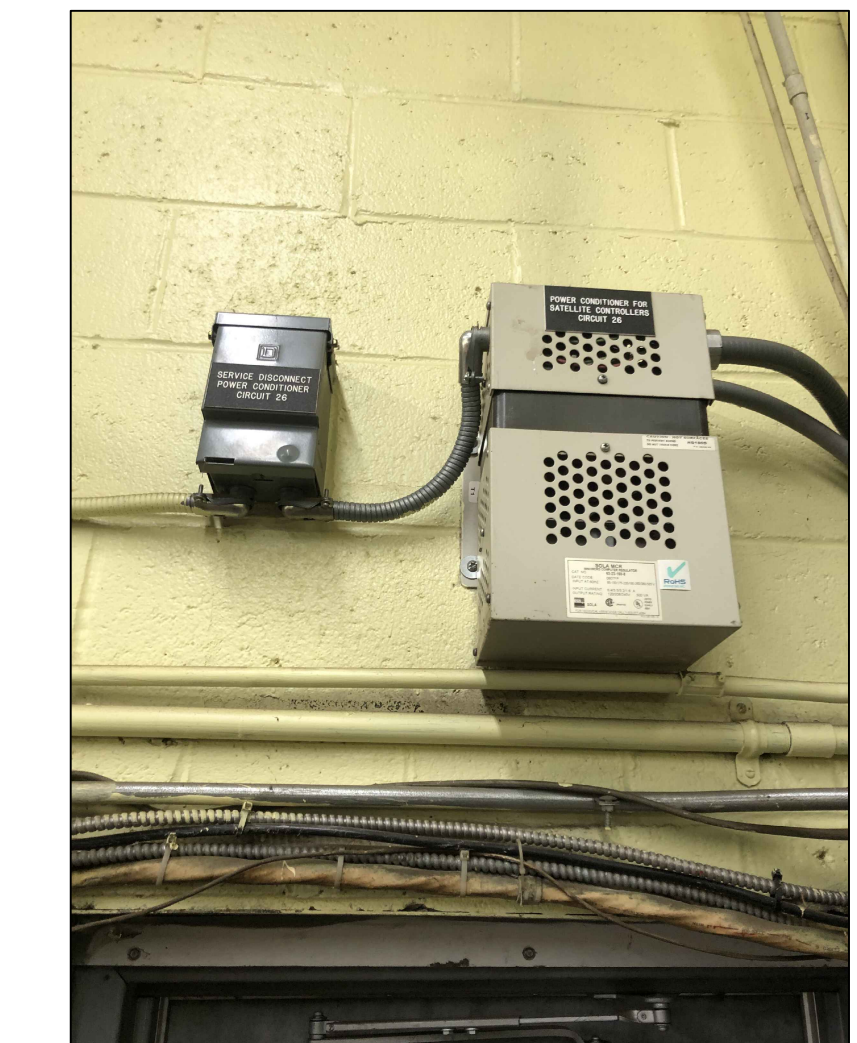
3 EXISTING IRRIGATION POWER CONDITIONER E2.0
