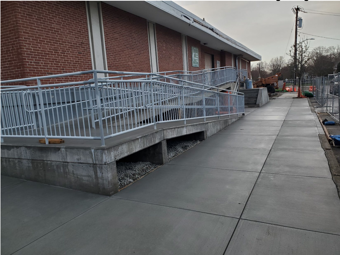
The new fully accessible main entrance to the Gath Pool bathhouse is substantially complete and we just poured the new sidewalks out front.
