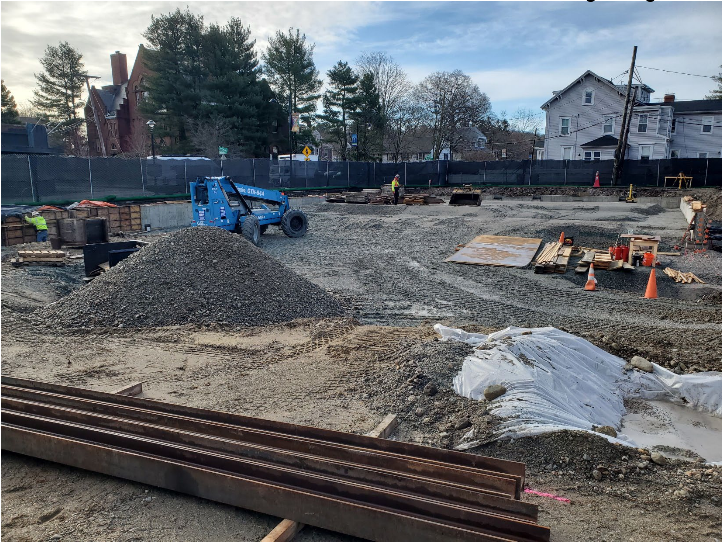
The bulk of the foundation has been poured now and the footprint of the building is starting to take shape.
