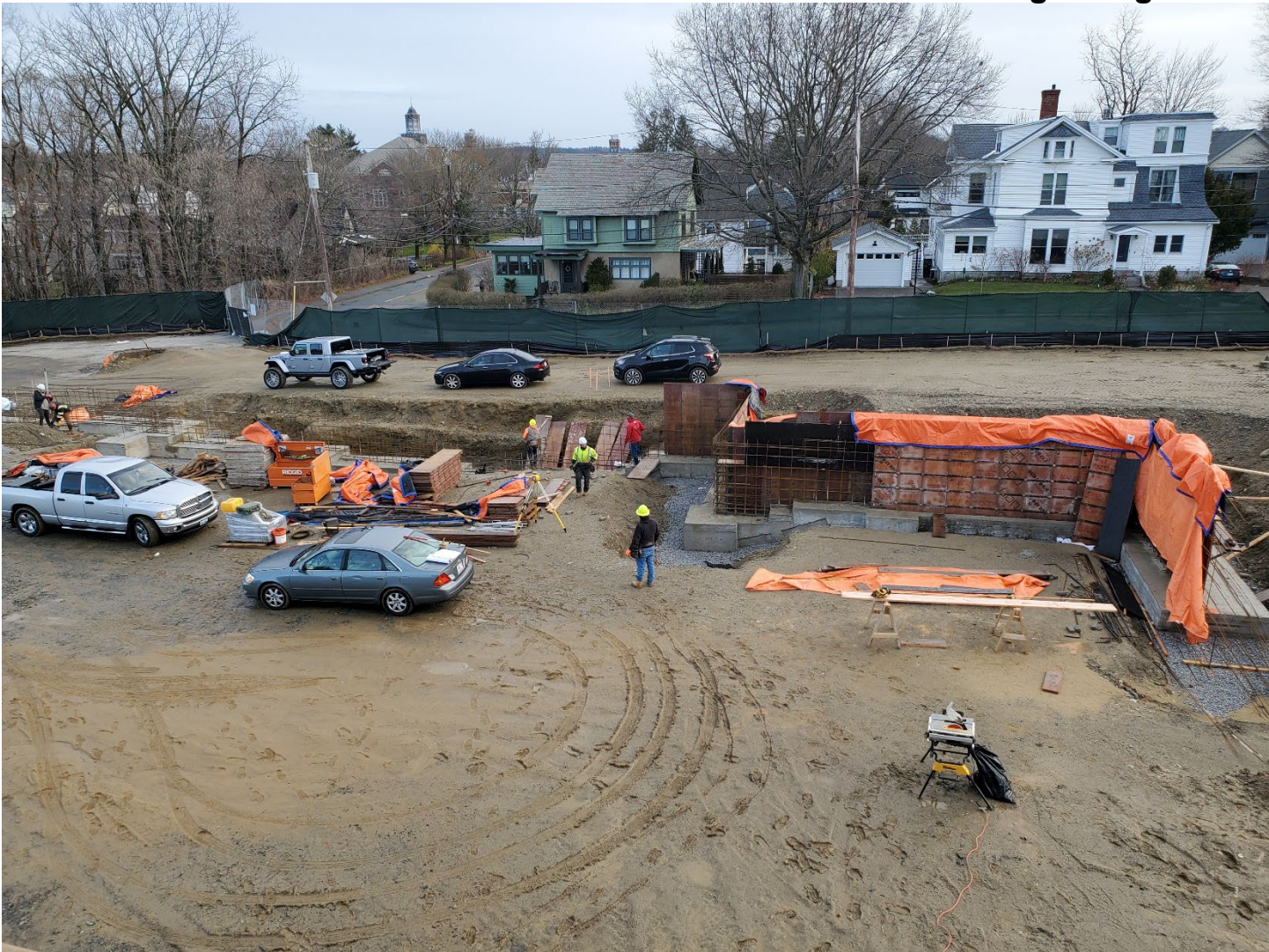
Outside, the crews are making short work of establishing our foundations for the new addition which will include the main entrance and office, the library, and the gymnasium.
