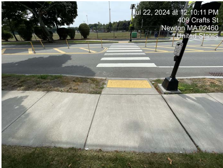
Crafts Street looking southerly toward the park, no sign of the manhole as shown on sheet C-100.
