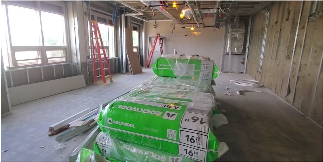
Inside the building, the crews from every trade are flying. Rockwool insulation and drywall are going up fast, so the spaces are really coming together.
