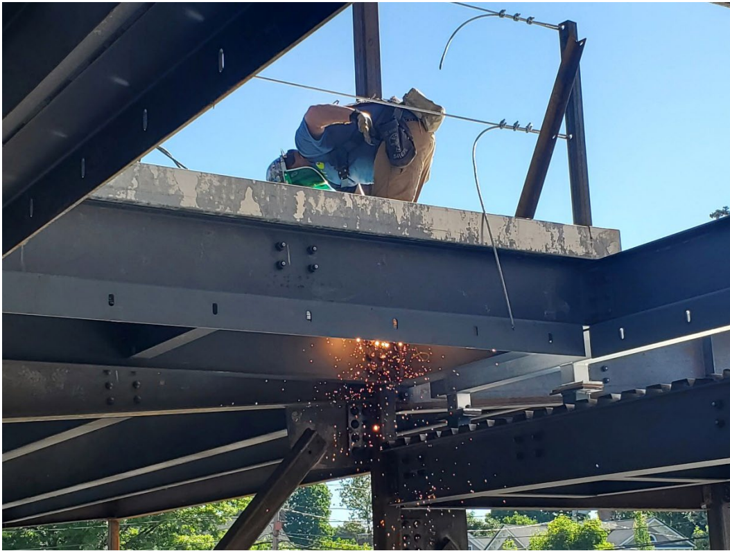
The steelworkers did a great job buttoning up the frame for the new addition.
