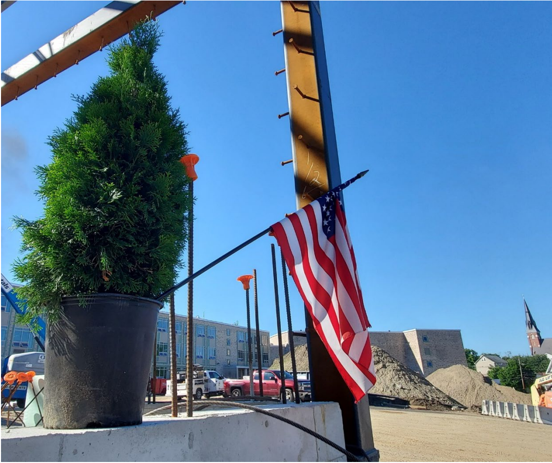
We had a great Topping Off Ceremony. The beam was signed by tons of Lincoln-Eliot students, parents, and staff, and it will be visible for generations to come inside the new gym.
