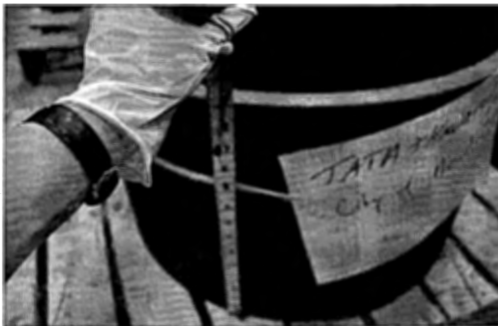
Figure 4: An overall view of a region of wall with corrosion from both ID and OD.
