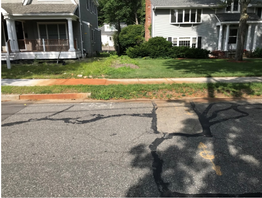
Overflow onto sidewalk and street Photo Taken July 16, 2019
