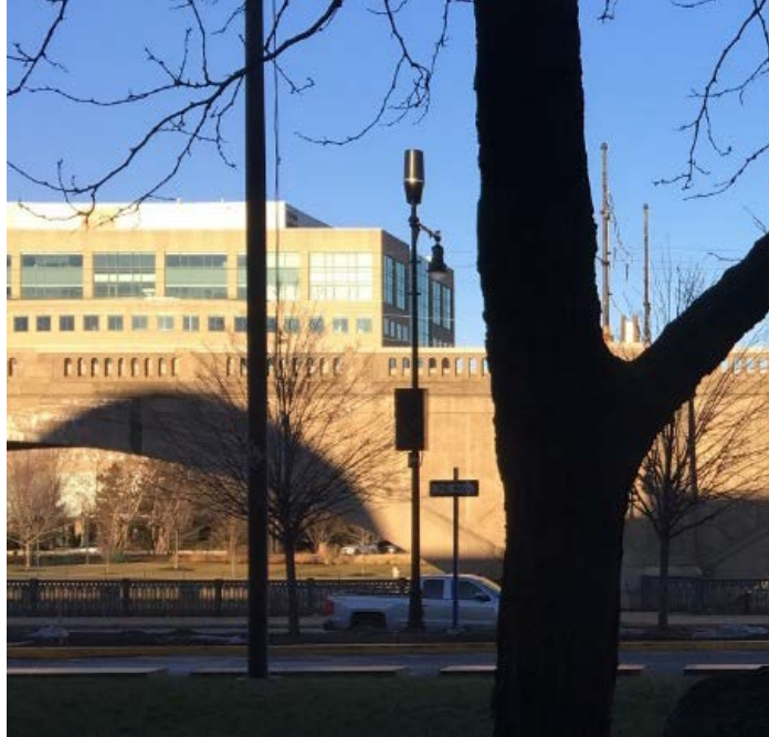
ABOVE: Example of wireless facility on a decorative pole, Museum of Science, Cambridge.
