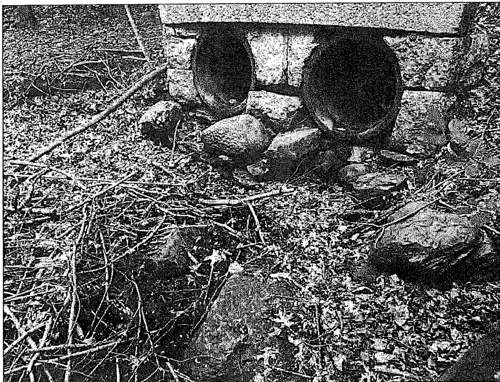
Photo No. 12: Low level outlet discharge headwall and standing water in the downstream channel.
