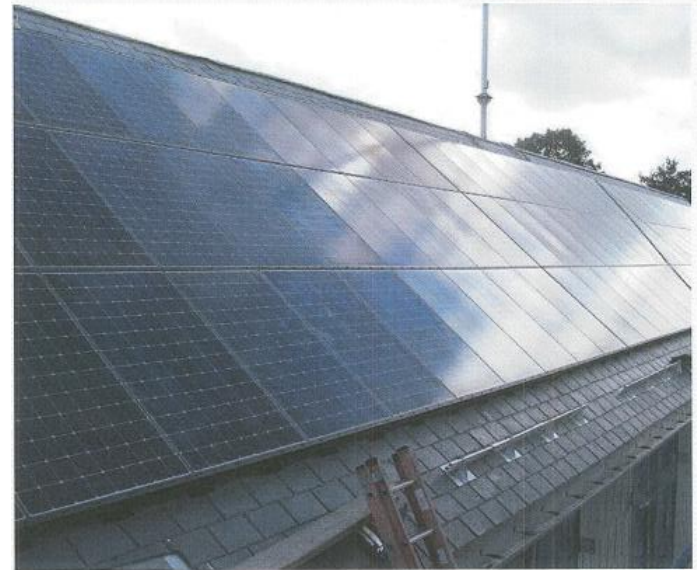
Perkins School For The Blind, Watertown, MA 33KW
