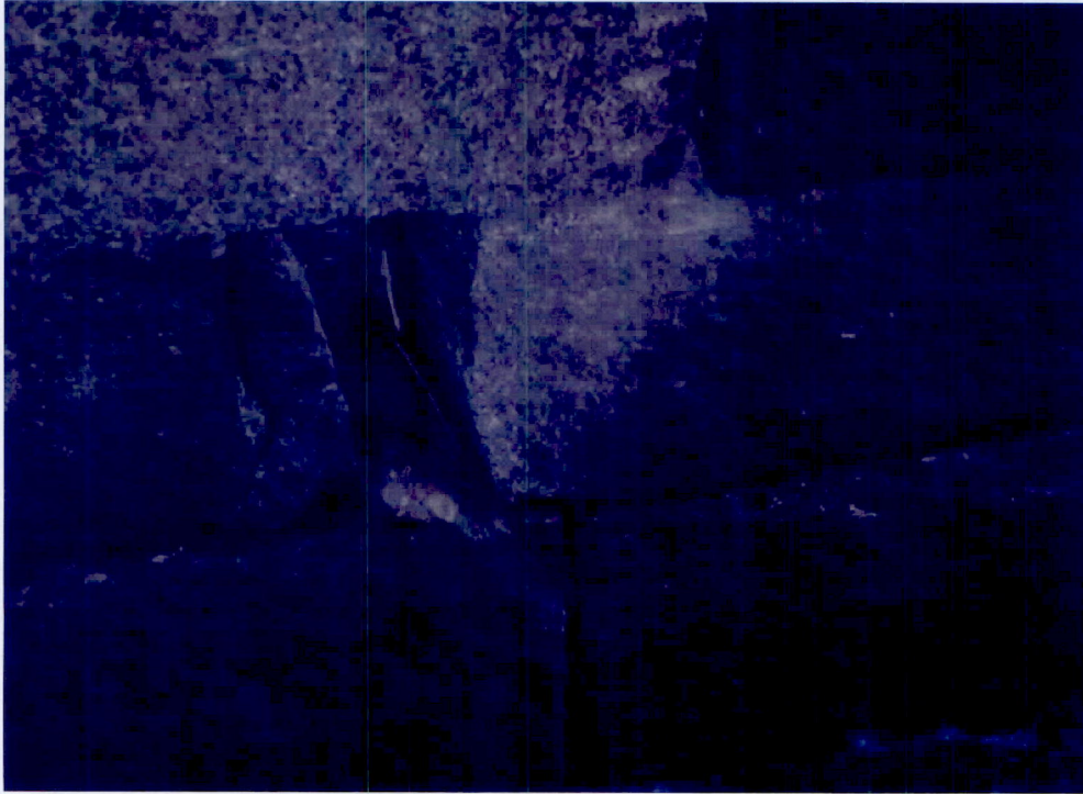
Photo 11: Split and void at north end of second block from the north at the second course above pier 2 springline in span 3.
