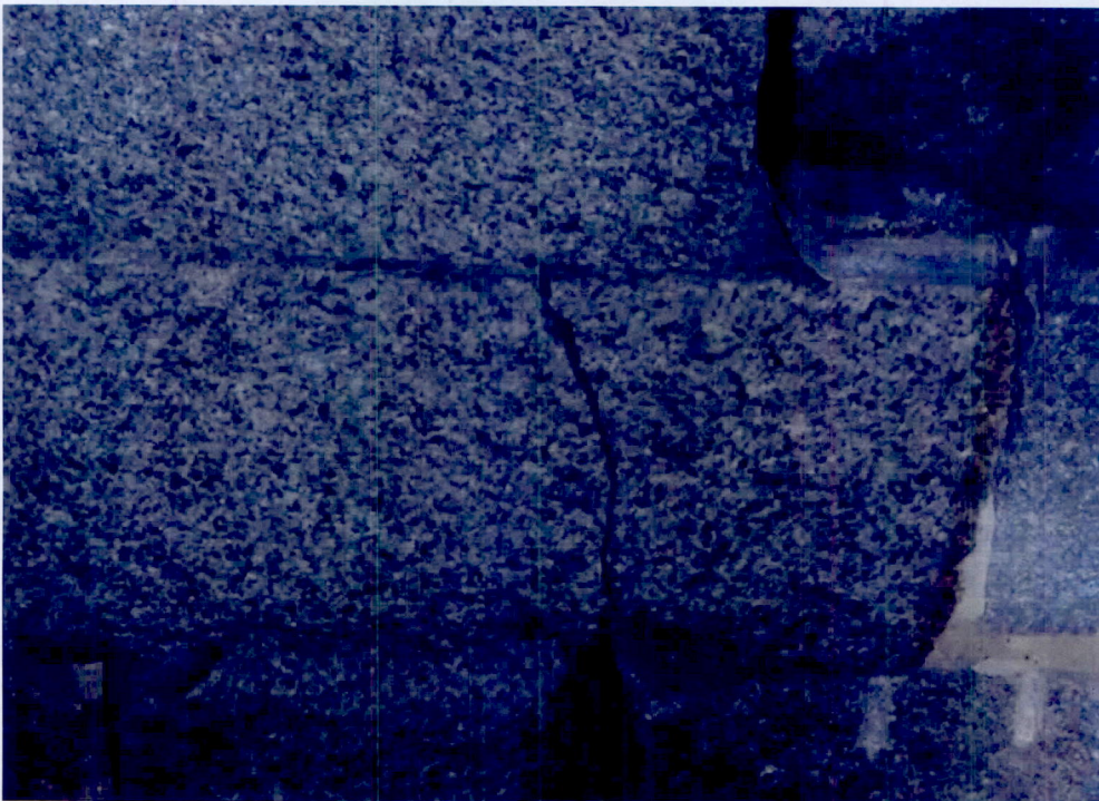
Photo 2: Span 1 split through seventh course of granite blocks above pier 1 at fourth block from the south.
