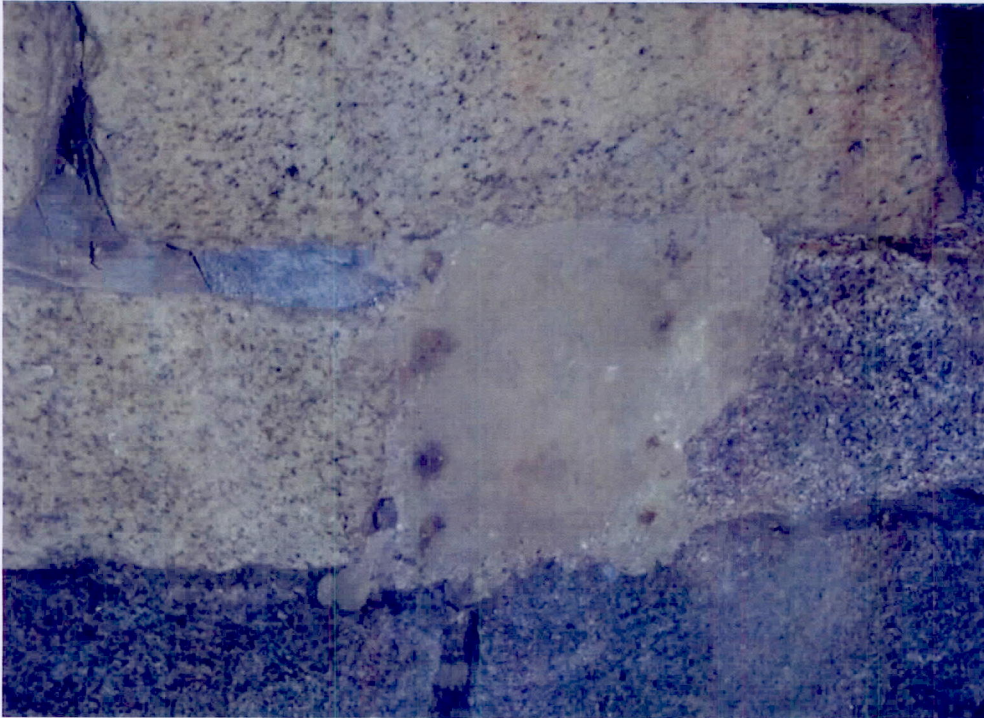
Photo 5: Concrete patch repair in span 2 just west of the keystone at the second block from the north.
