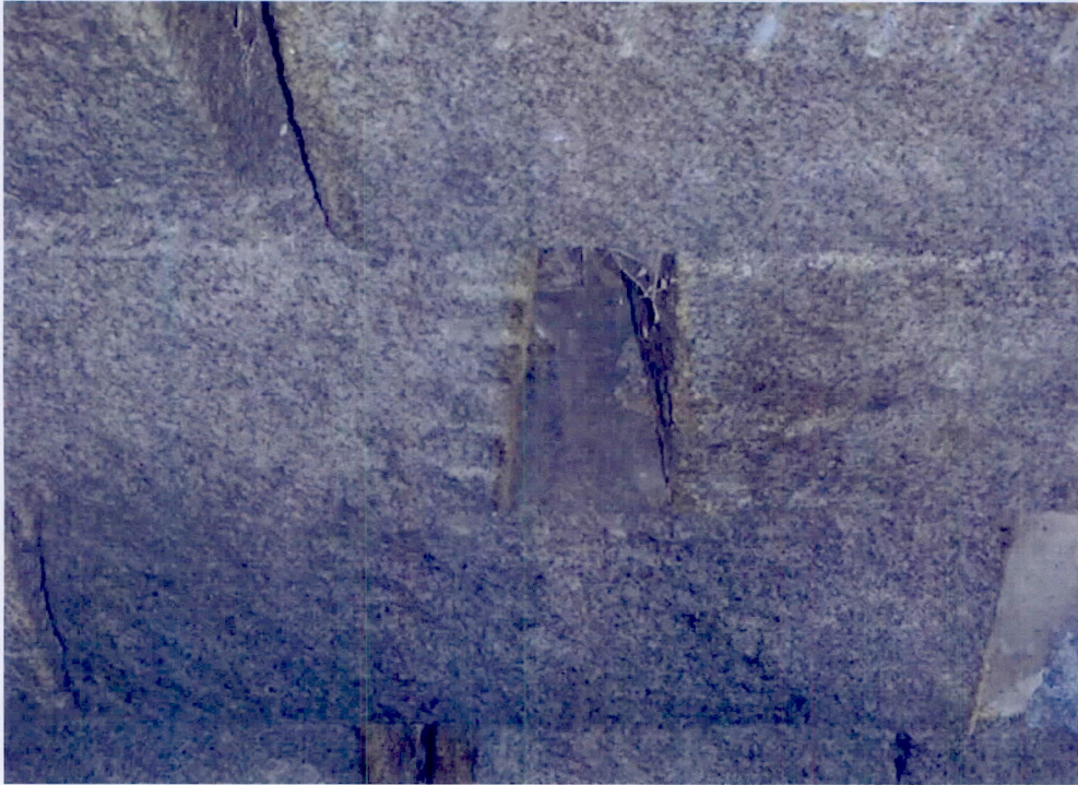
Photo 3: Void up to 8 1/2" wide between the fifth and sixth granite blocks from the south at second course east of keystone in span 1.
