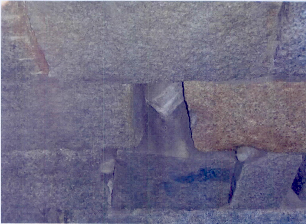
Photo 9: Voids at the fourth block from the north at the sixth and seventh course above pier 1 springline in span 2.
