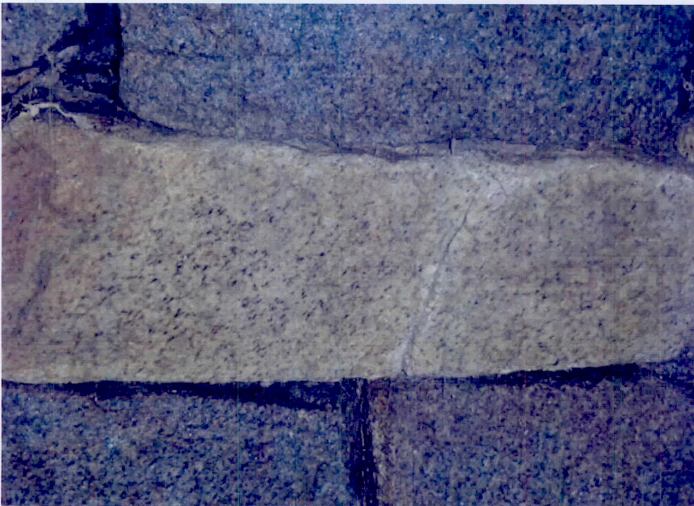
Photo 6: Through crack, first course east of keystone at the third block from the north in span 2.
