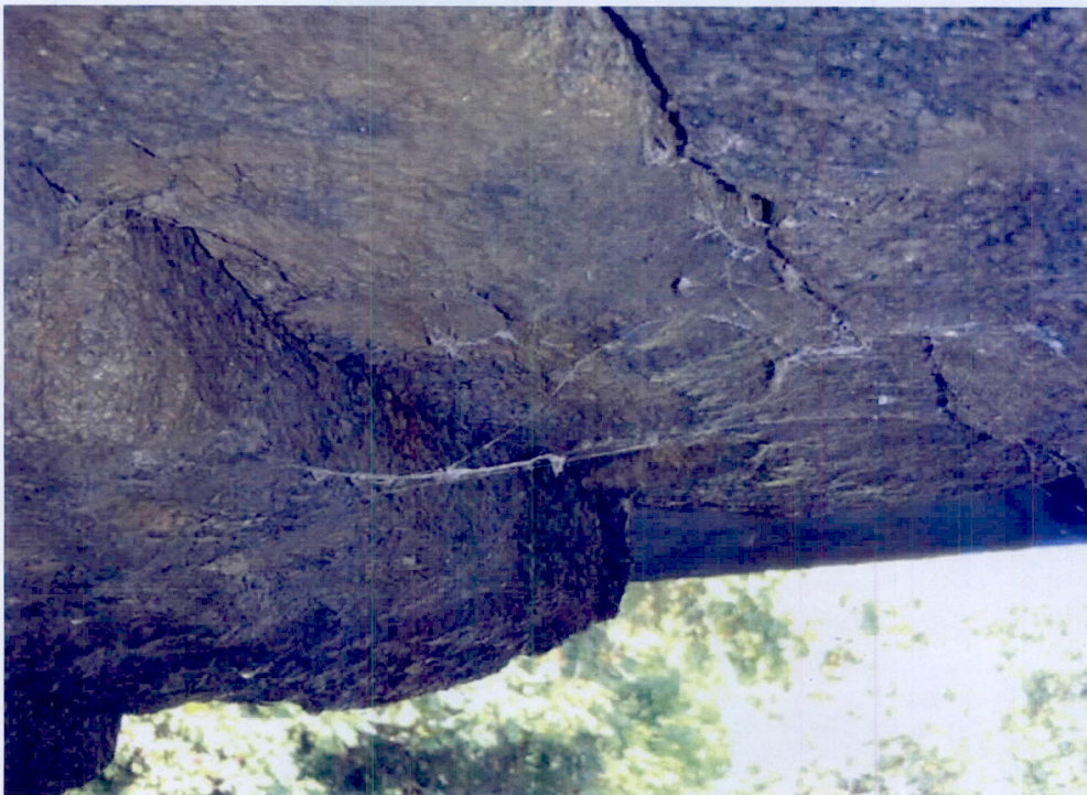
Photo 12: Keystone 3" higher than adjacent blocks at north end of span 3.
