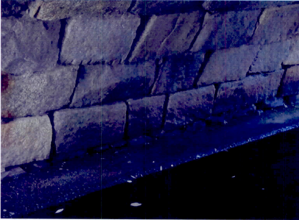
Photo 17: Span 2, top of pier 1 east face, cracked stones.
