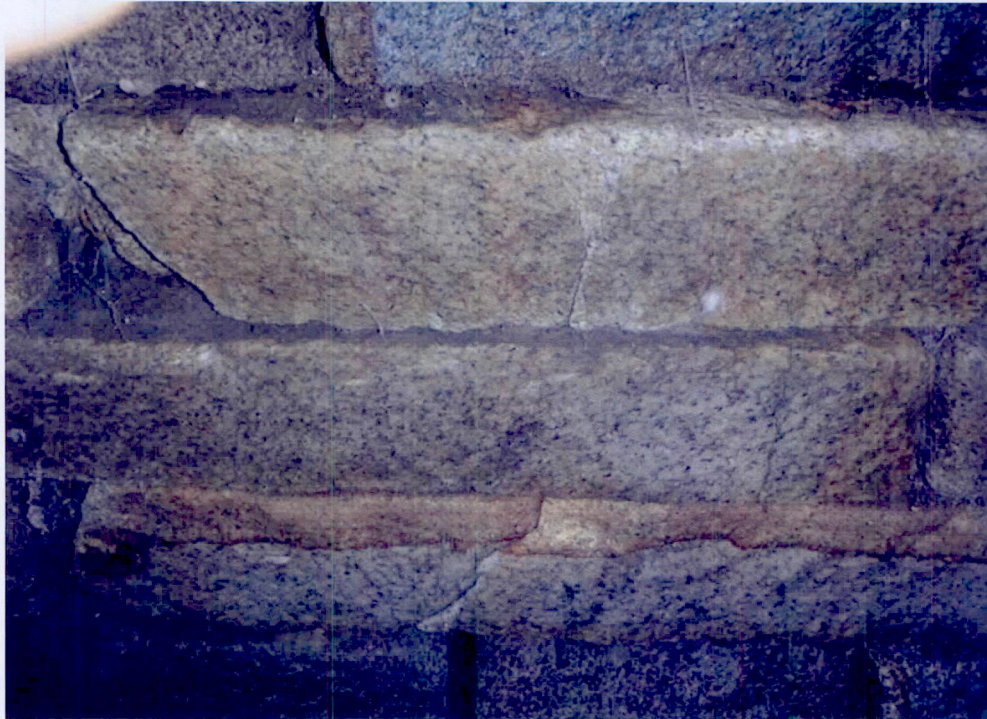
Photo 7: Cracked granite in first and third blocks west of keystone at fourth and fifth blocks from the north in span 2.
