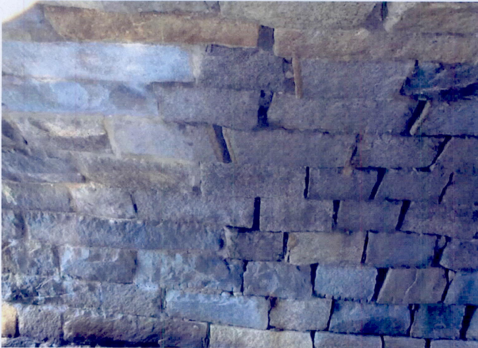
Photo 1: Separation along masonry joints at connection of original arch to widened section of arch in span 2.
