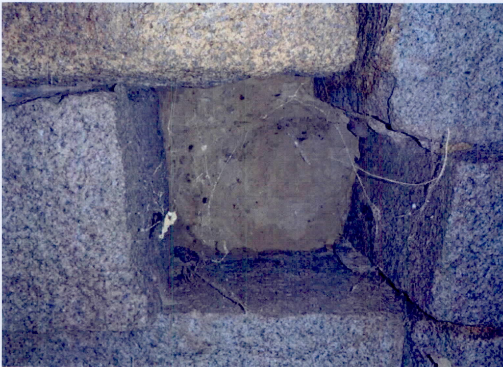
Photo 10: Span 3 fourth block from the north just east of keystone, missing block, 17" W x 19-1/2" L x 2' D.
