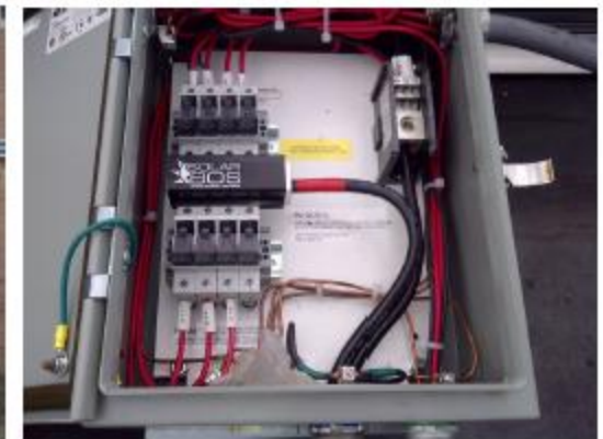
Commissioning & Witness Test
