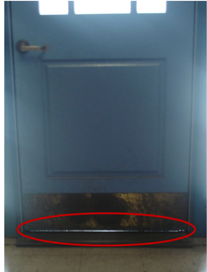
Unsealed Door Jamb at Police Headquarters
