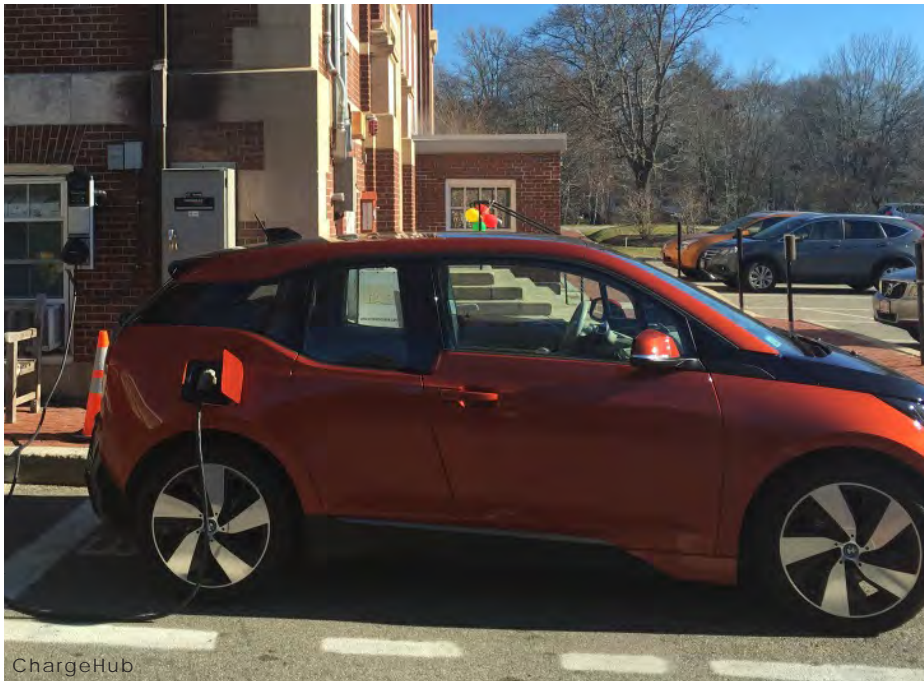
EV-charging is available at City Hall and becoming more common at residences and offices.
