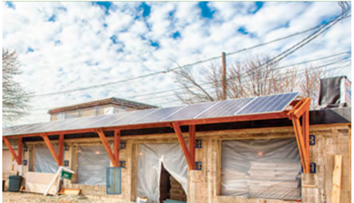
Auburndale Builders is retrofitting an existing office building to meet Passive House standards on Adams Street.
