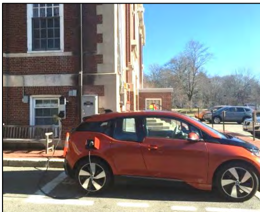
Clean vehicles: City Hall EV charging station
