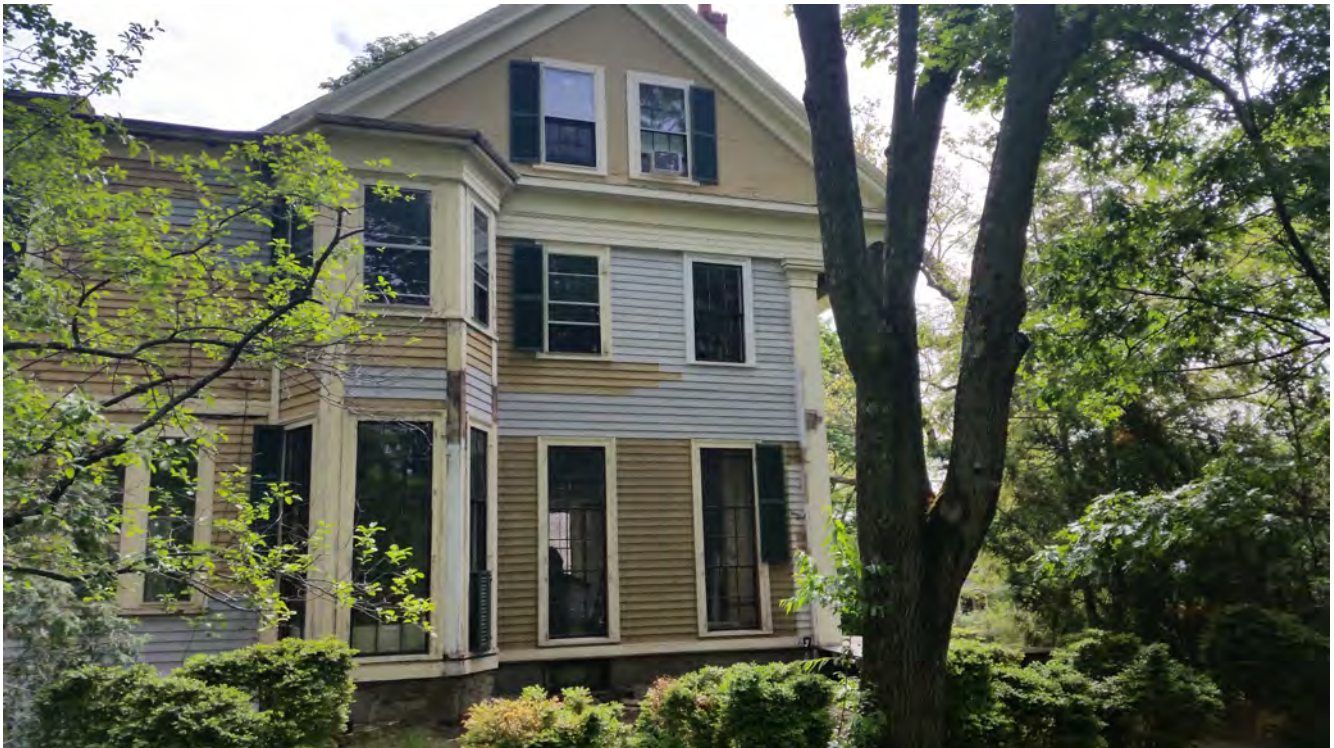
CPC Phase I work: Cherry St. façade work completed—porch demo, new window & siding
