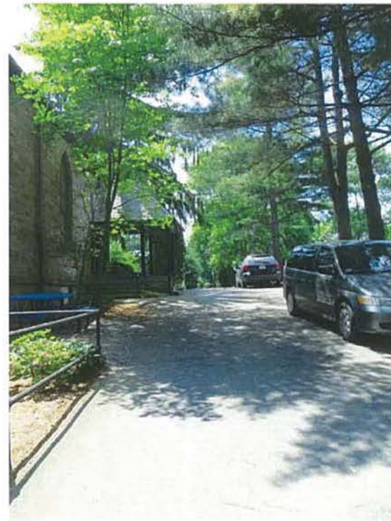
Figure 9: Driveway which needs to be repaved
