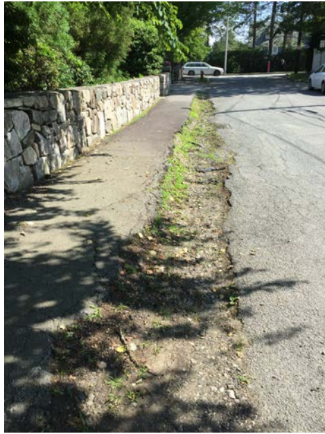
Pavement derogation due to a lack of curbing
