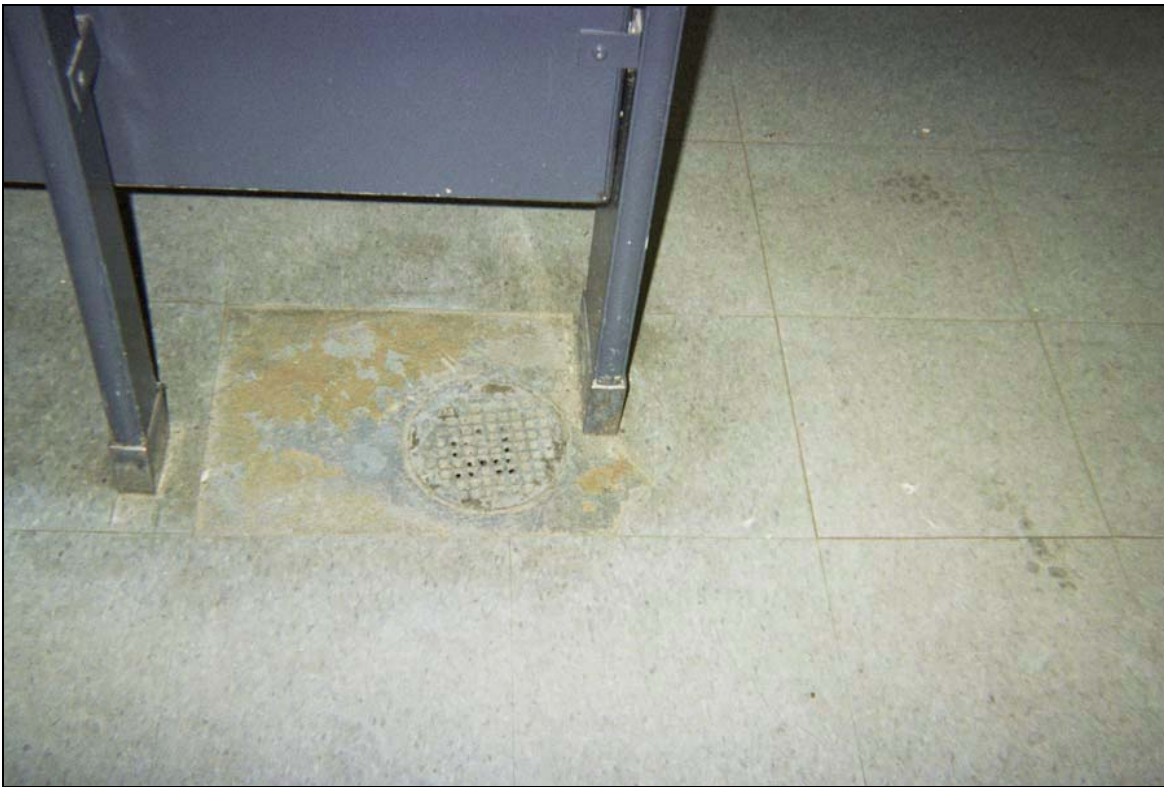
Figure 23: Interior Bathhouse - Single Floor Drain
