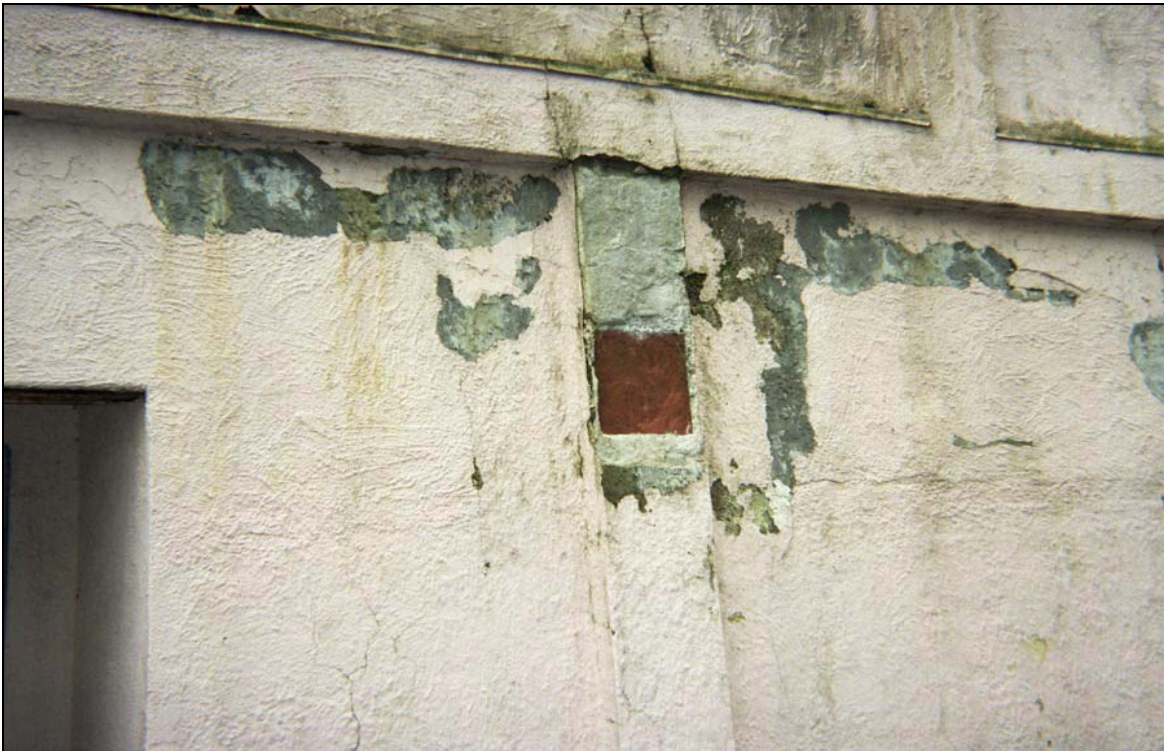
Figure 17: Exterior Bathhouse Wall - Stucco Over Clay Tile
