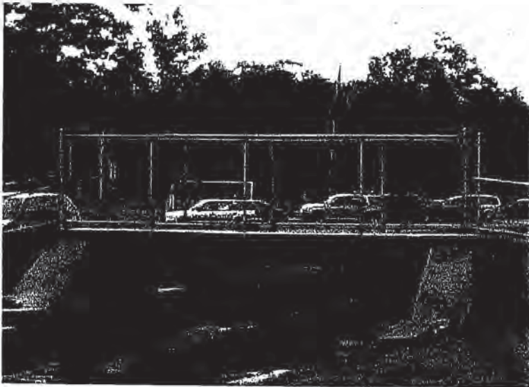
The foot bridge over Cheesecake Brook. This is the only footbridge connecting the two lanes of Albemarle Road
