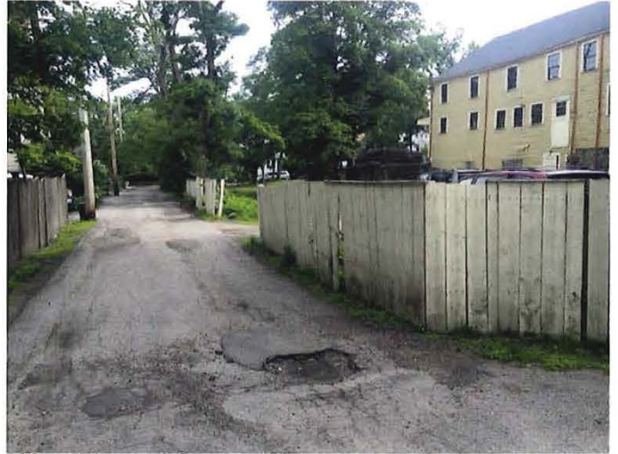
Wood board fence along Eastern property line
