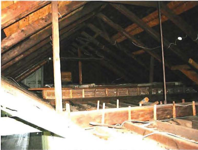
Heavy timber roof trusses with iron rods in place of king posts above Gymnasium
