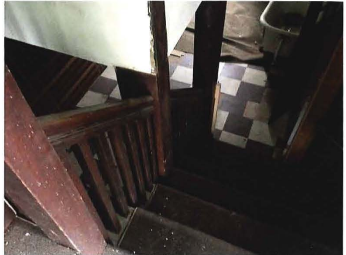
Entrance Hall and Stairway newell post, handrails and balusters
