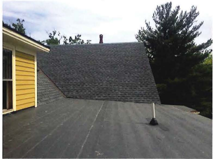
North side asphalt roof of Main Block, West Side Ell flat roof and dormer
