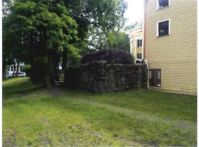
Columbus Place full story retaining wall at the Southeast corner of the Barn
