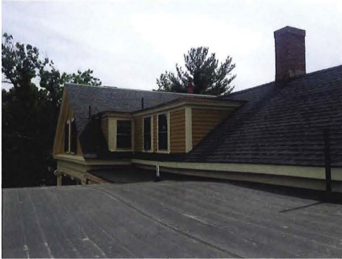
North side asphalt roof and dormer of Main Block. Rear Ell asphalt roof, dormers and chimney. East Side Ell flat roof.
