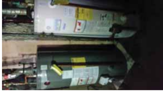
Basement – Two Water Heaters
