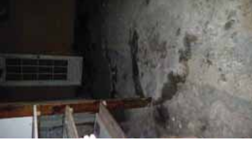
Basement – Water Staining
