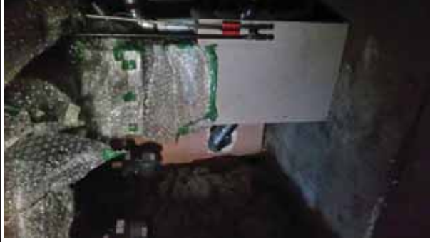
Basement – Gas Furnace #2
