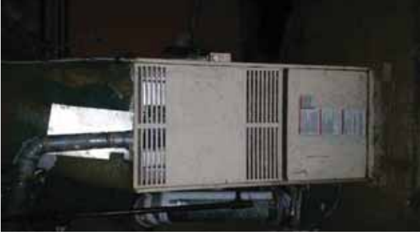
Basement – Gas Furnace #4
