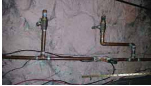
Interior – Basement Plumbing
