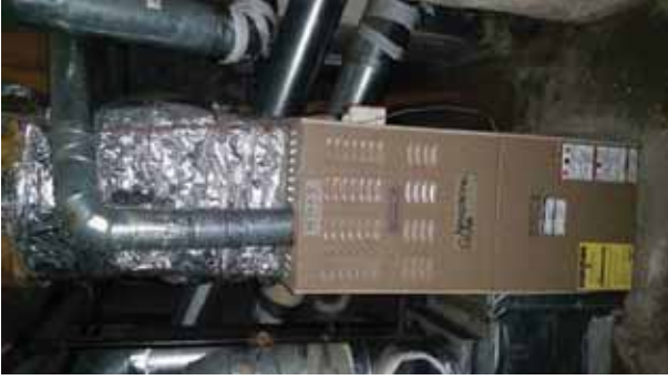
Basement – Gas Furnace #3
