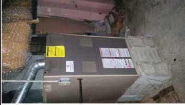
Basement – Gas Furnace #1
