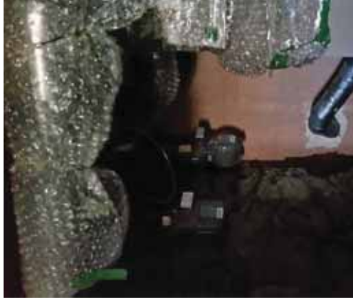
Basement – Gas Meters
