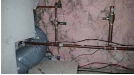
Interior Basement Plumbing
