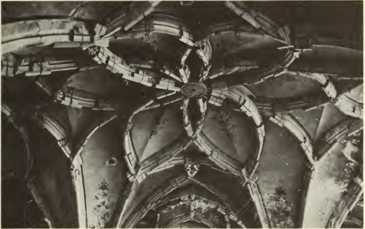
Figure 17: This photograph further illustrates the elaborate measures taken to stabilize the structure. The groins of the intricately detailed lierne vaulting were braced to cushion them from possible shocks during moving, and to make certain that this area of the church was tied into the monitoring system. [Photograph from a slide by Jack E. Boucher, 1975]
