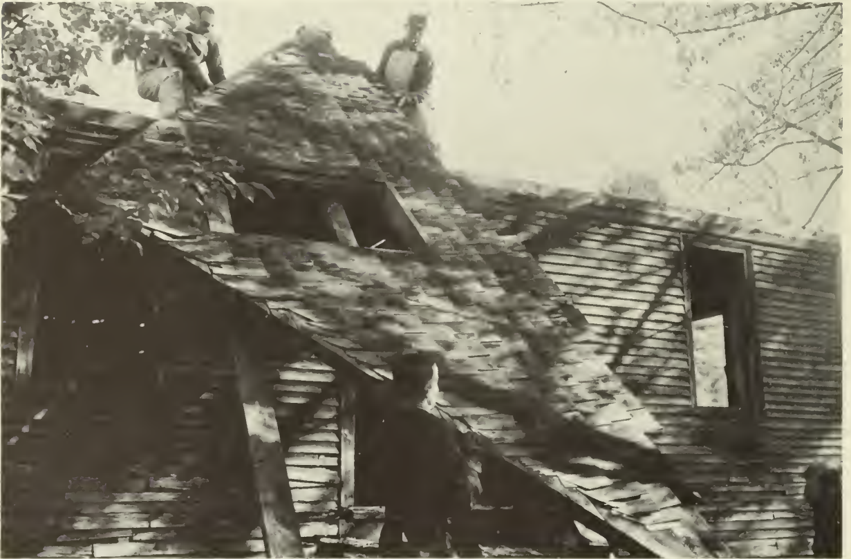
Figure 24: The entire gable end of the Hapgood Carding Mill is handled as a unit in a partial disassembly. [Photograph: John O. Curtis, Old Sturbridge Village]
