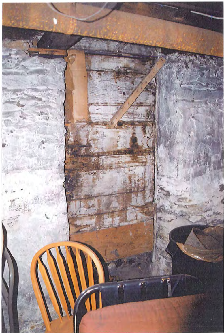
BASEMENT - ROTTED WOOD
