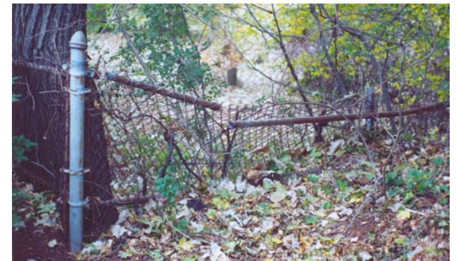
collapsed chain link fence, South Burying Ground
