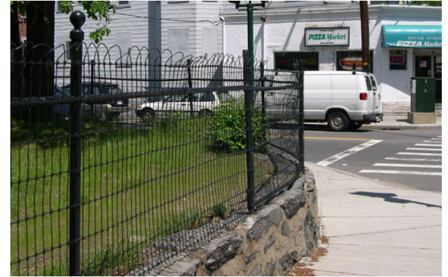
damaged crosslink fence - West Parish Burying Ground
