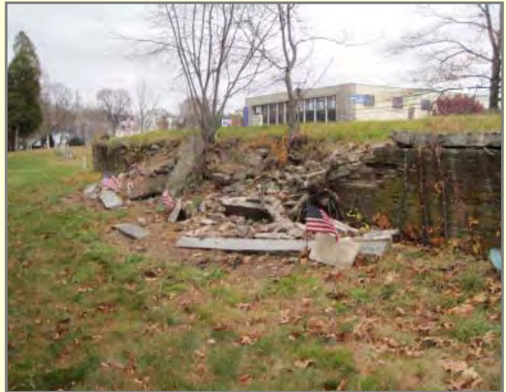
Collapsed tomb wall at South
