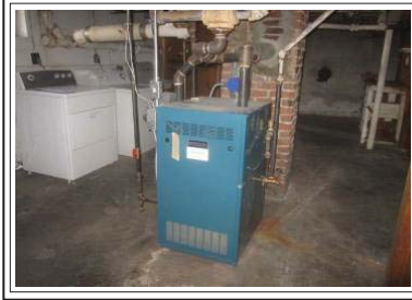
HEATING SYSTEM UNIT#1 AND UNIT#2
