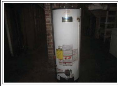
WATER HEATER IN THE BASEMENT
