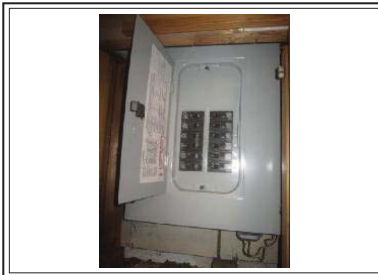
ELECTRICAL BOX IN THE BASEMENT
