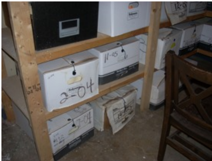
Record cartons stored in the room on the second floor of City Hall behind the Aldermanic Chambers show evidence of past water damage.
