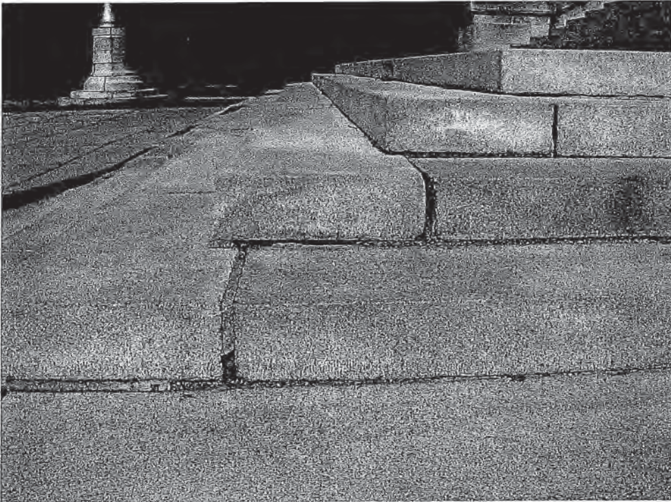
Photo D - Damage & Displacement of Stair Treads at South Side of Stair
