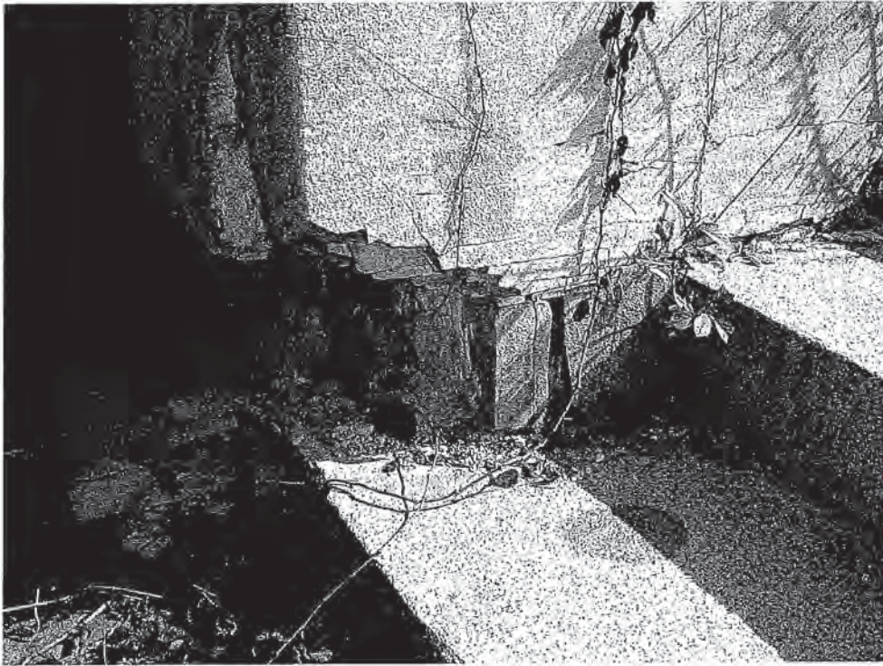
Photo C - Limestone Disintegration at Base of North Stair
