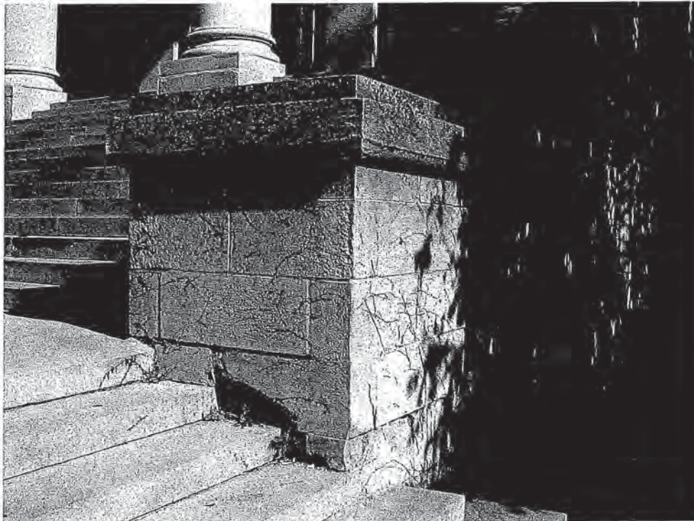
Photo B – Limestone Disintegration at Base of South Stair
