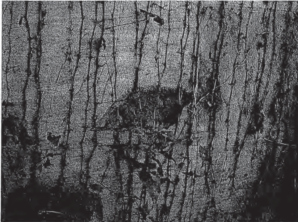
Photo F - Spalling of Stone Facing at Walls
