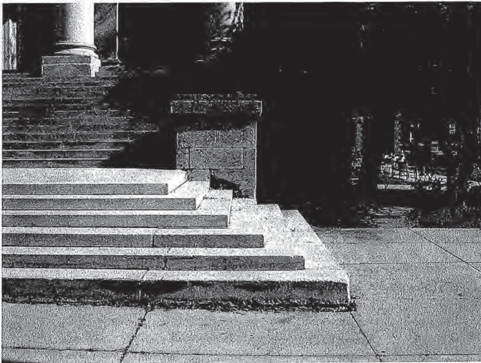
Photo A – View of South Stair Wall and Stair Showing Pier and Treads
