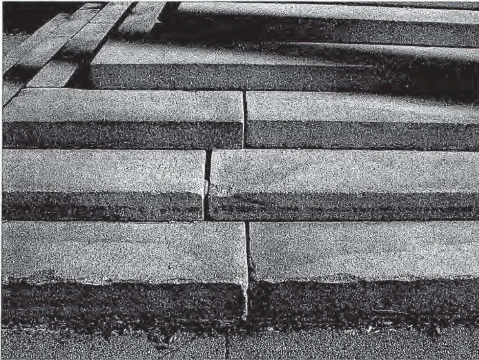
Photo E - Damage & Displacement of Stair Treads at North Side of Stair
