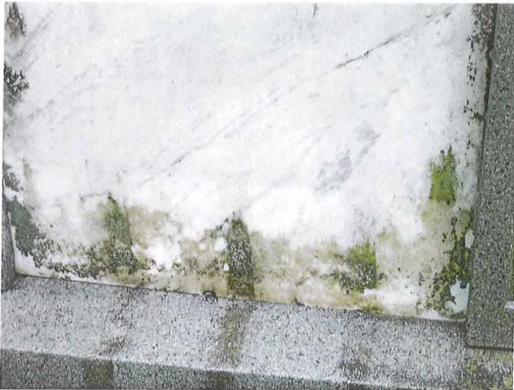
Newton Cemetery Civil War Memorial : Heavy biologic soiling. From left to right: Light Duty Restoration Cleaner, Klenztone #2 (best result), Bac2Nu, Diedrich 910 Marble Cleaner.
