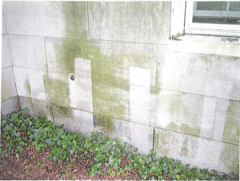
Newton City Hall War Memorial : Limestone and granite in testing area. From left to right: Powerwash with water, Bac2Nu, Klenztone #1 (best result), Light Duty Restoration Cleaner.
