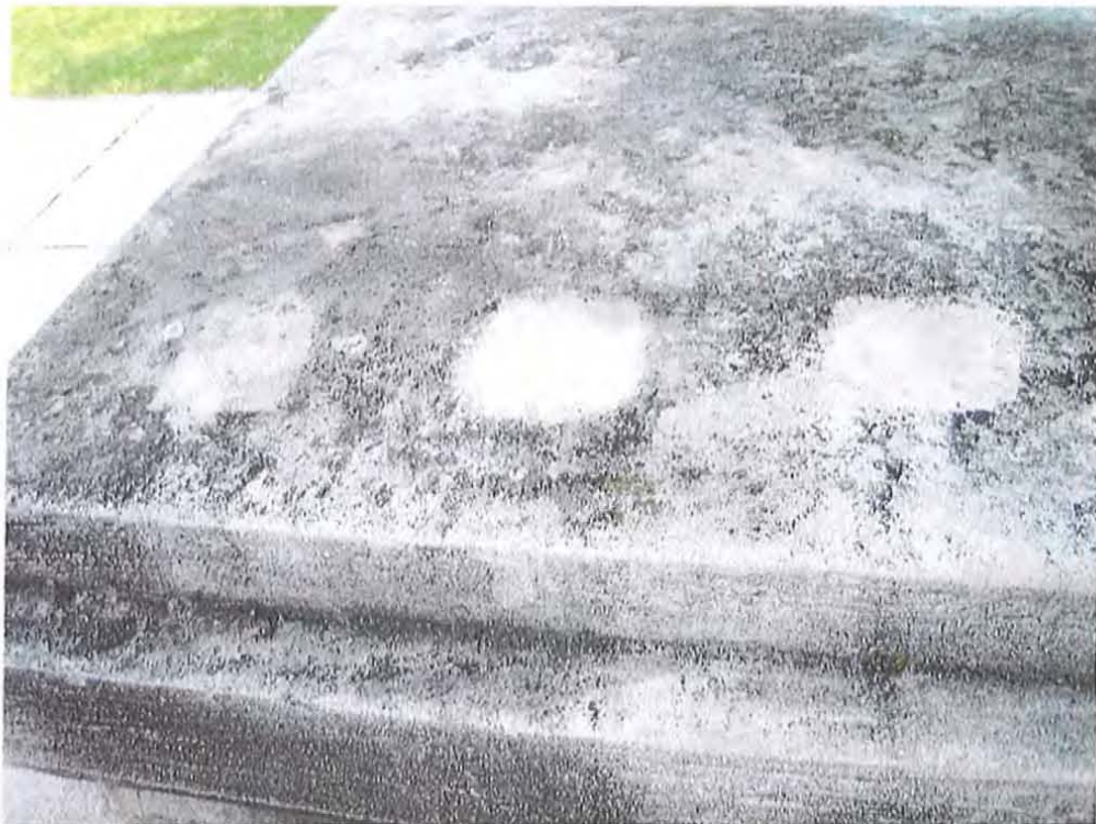
Newton City Hall War Memorial : North pier at steps. Heavy biologic soiling. From left to right: Powerwash with water, Bac2Nu, Klenztone #1 (best result).
