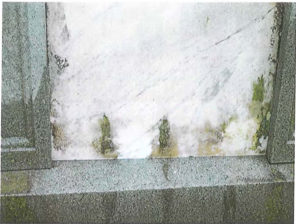
Newton Cemetery Civil War Memorial : From left to right: Prosoco 1260 , Sodium Hypochlorite (best result), T-1087, Hydrogen Peroxide, Prosoco 942 (not pictured here).
