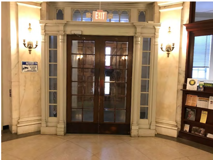
Interior Door Not Accessible
