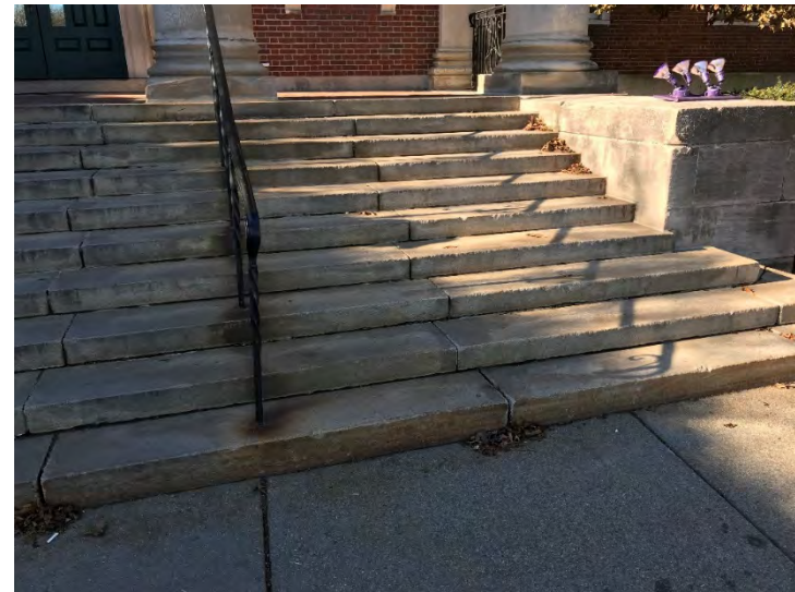
Open Joints on the Right side of the Stairs and Buttress
