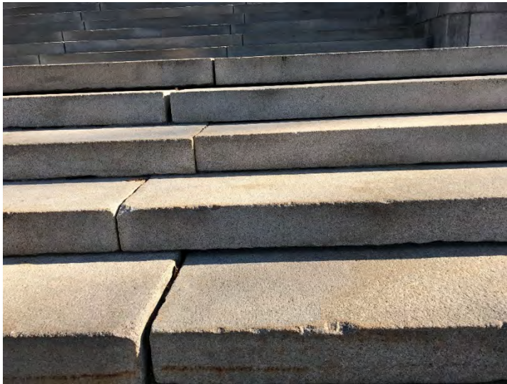
Open Joints and Settlement of the steps
