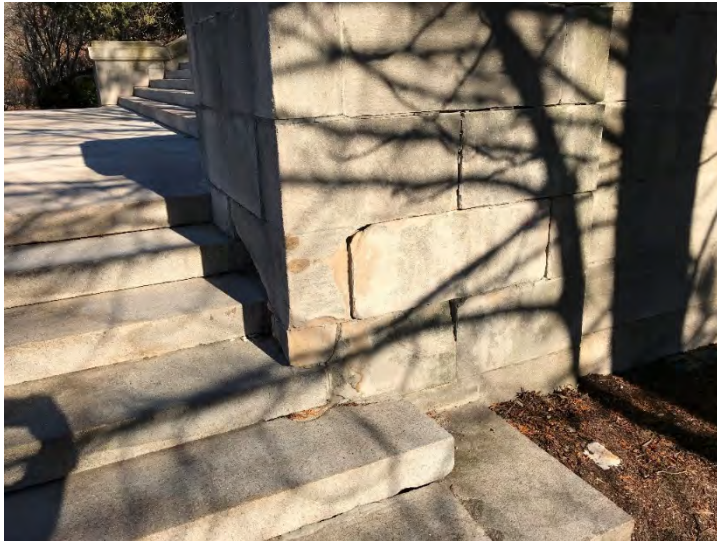
Open Joints at Stairs Buttress
