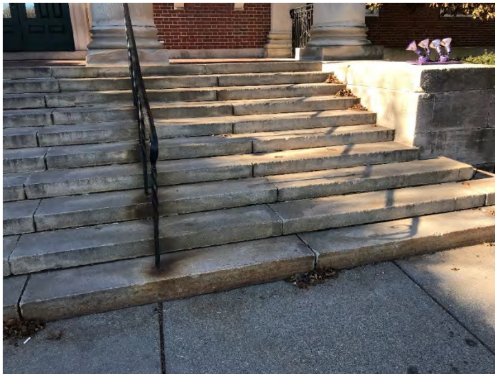
Deteriorated Joints and the Rail is Not to Code
