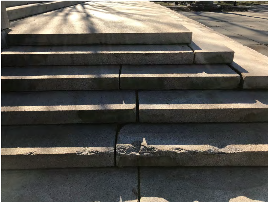
Open Joints and Steps Movement (Left Side)
