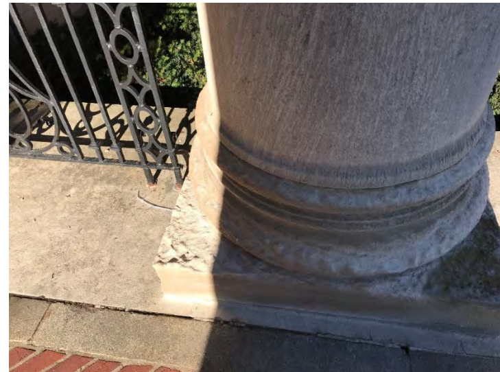
Deterioration at Column and Base
