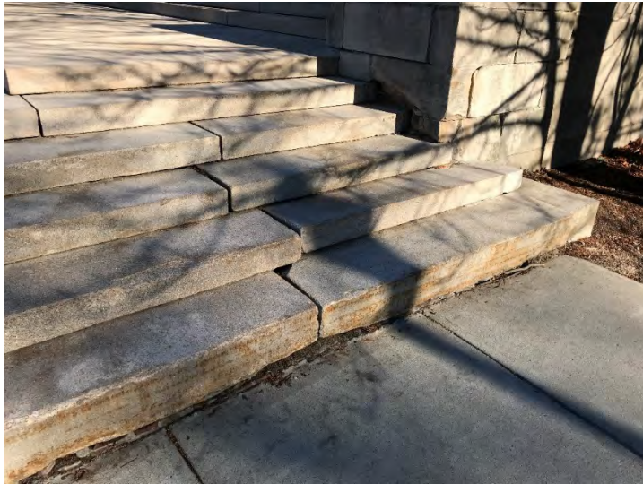
Steps and Concrete plaza settlement (right side)
