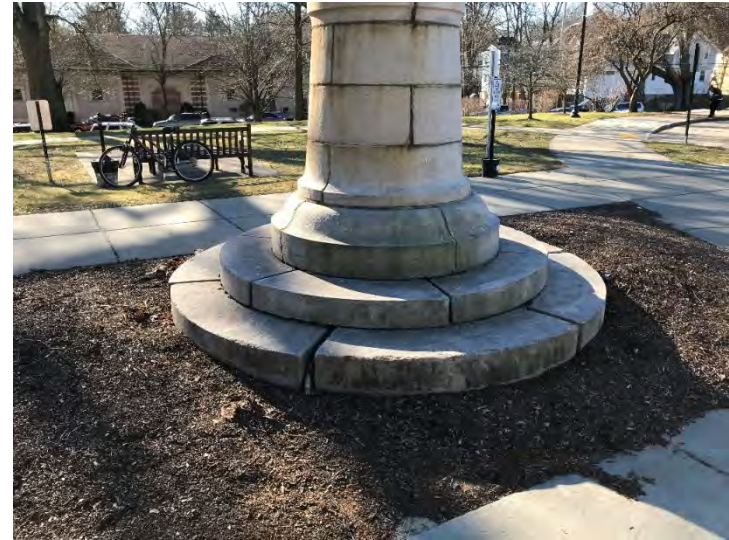
Right side Flag Pole Base deterioration
