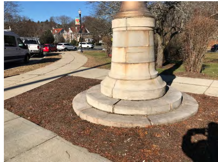
Left Side Flag Pole Base deterioration
