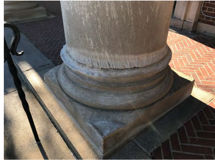
Deterioration at Column and Base
