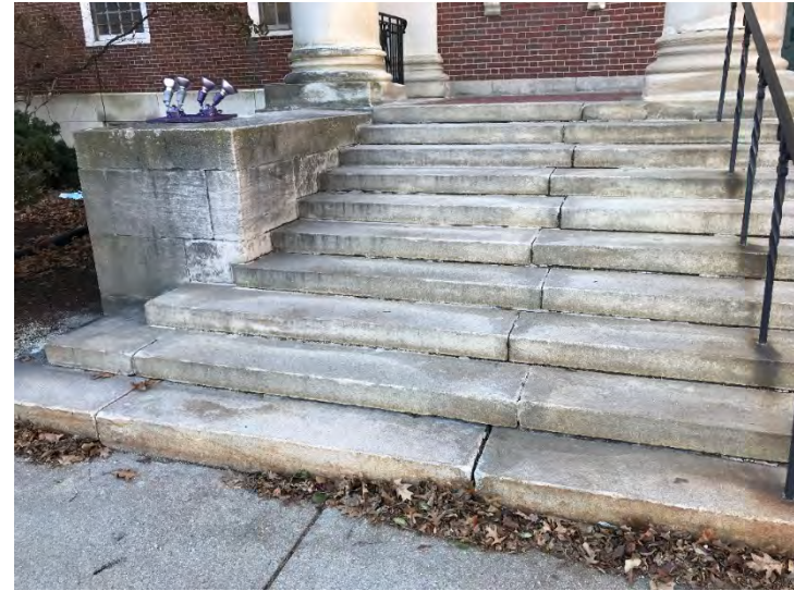
Open Joints on the left side of the Stairs and Buttress
