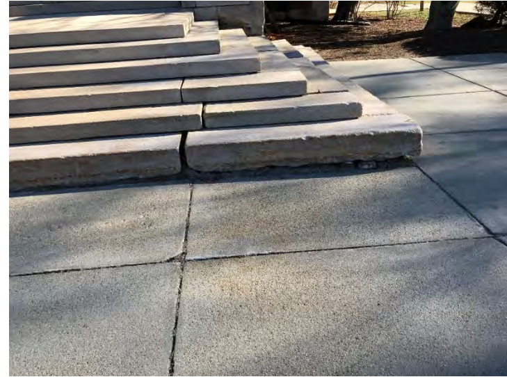
Concrete Plaza Settlement Causing First Step to Be Higher and Unsafe
