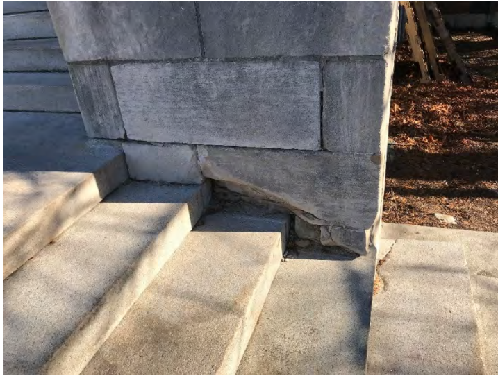
Limestone Deterioration at The Stairs Buttress
