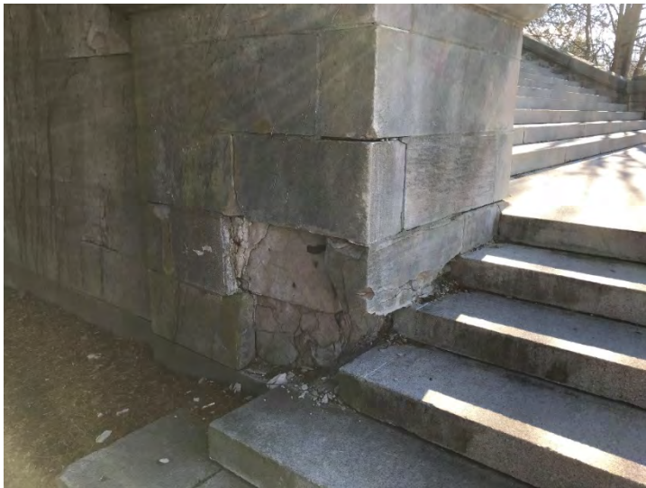
Limestone Deterioration at Buttress on the left side
