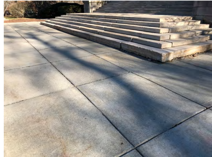
General View of Plaza settlement and Unsafe Steps
