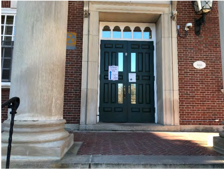
Entrance and Door Not Accessible
