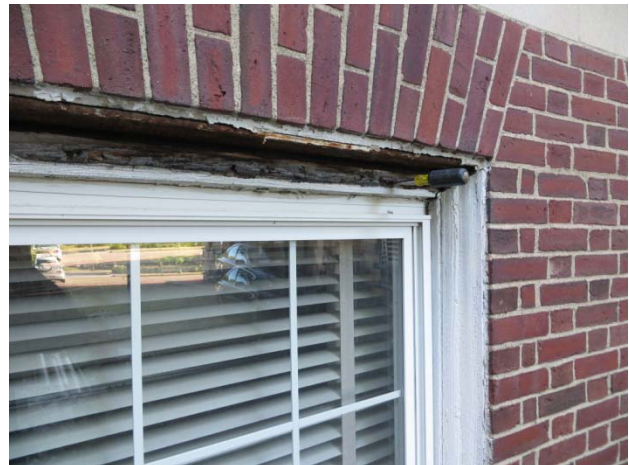
Missing head of frame and deteriorated steel lintel. Note missing flashing at lintel.
