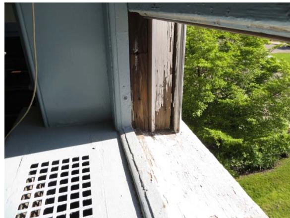
Jamb of typical window. No weather stripping installed at jamb or sill.
