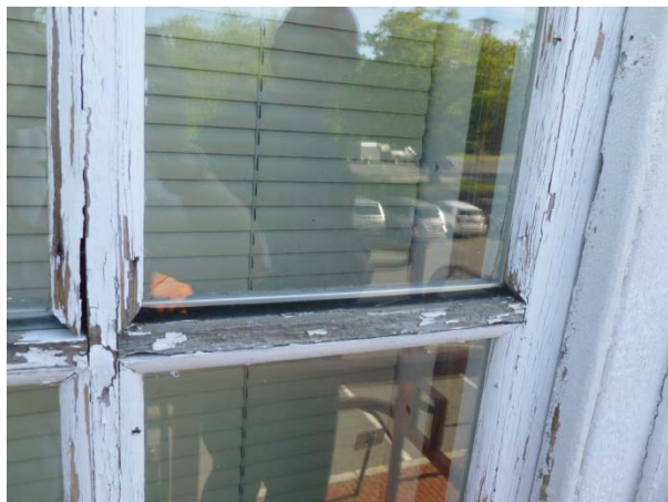
Missing wood stop.
