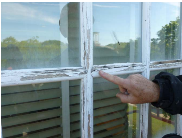
Failed paint at muntins and wood stops. Rusted brads sticking up out of wood.
