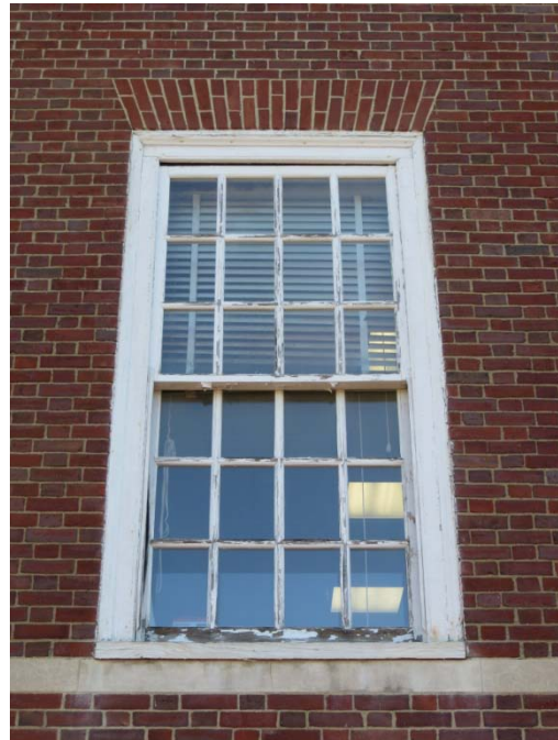
Typical retrofitted window with failed paint and failing wood stops.
