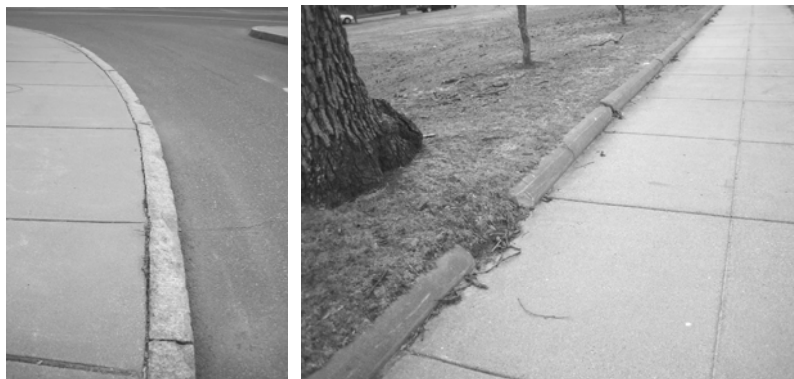
Figure 5.4. Granite and concrete curbs in need of repair or replacement, 2006 (Pressley Associates).
