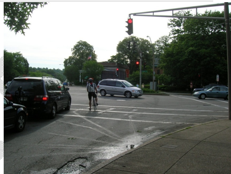
Figure 4. Centre St at Beacon St looking East - Potholes at southeast corner
