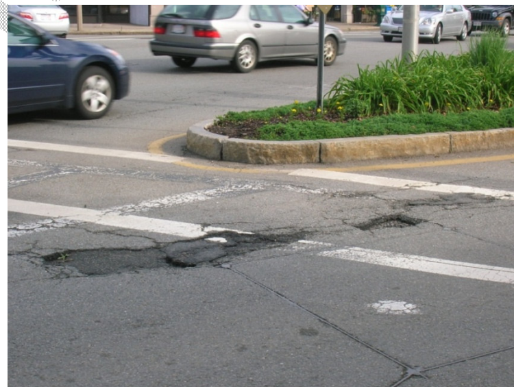
Figure 5. Centre St at Beacon St looking South - Potholes at southwest corner
