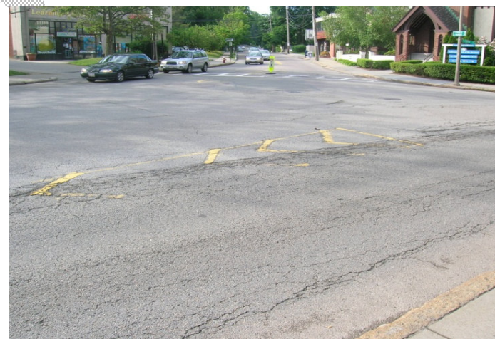
Figure 36. Centre St at Cypress St looking Southwest - Fading Pavement Markings
