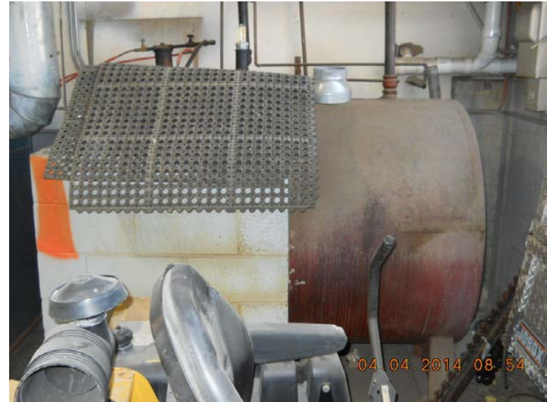
Photo #6: Fuel oil AST in garage
