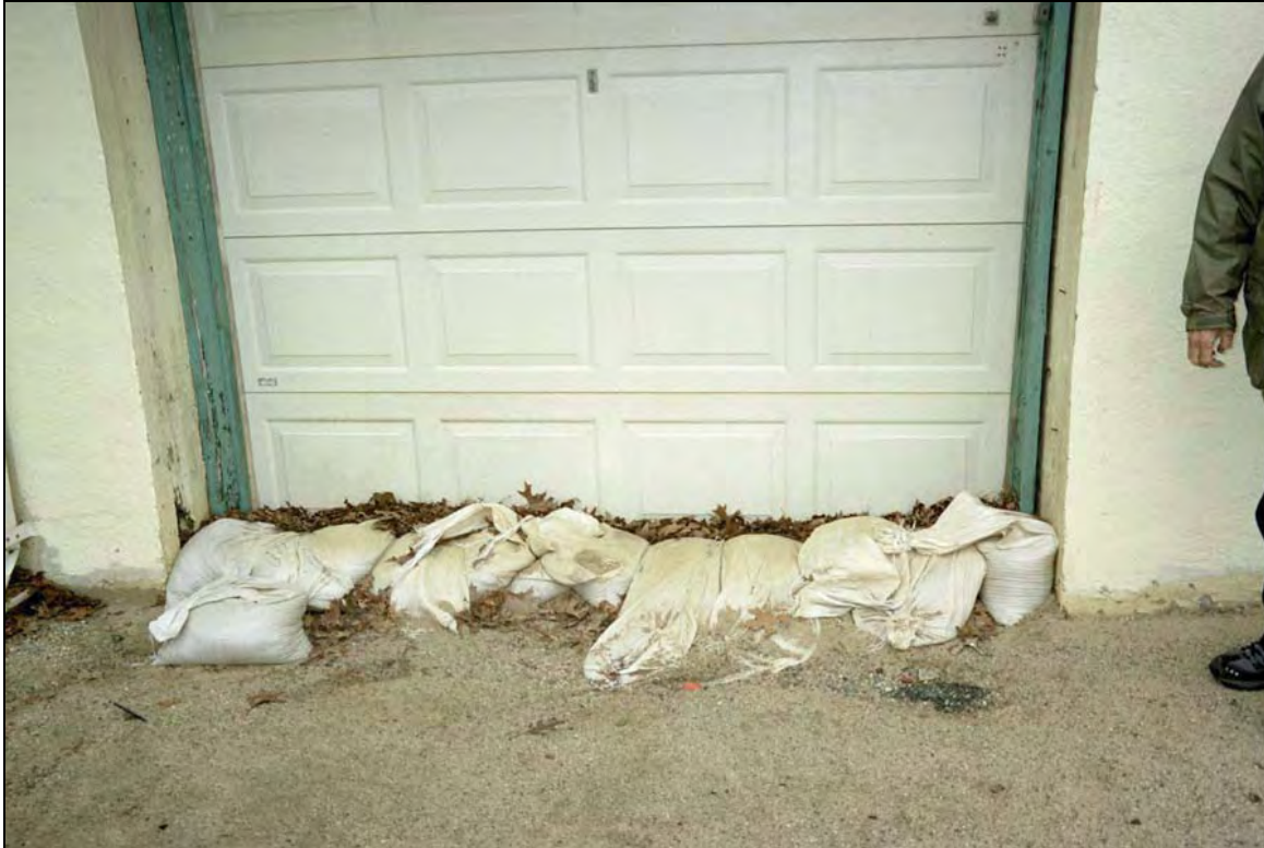
Figure 14: Exterior Bathhouse Lower Level Guardroom Door-Sandbags to Prevent Flooding
