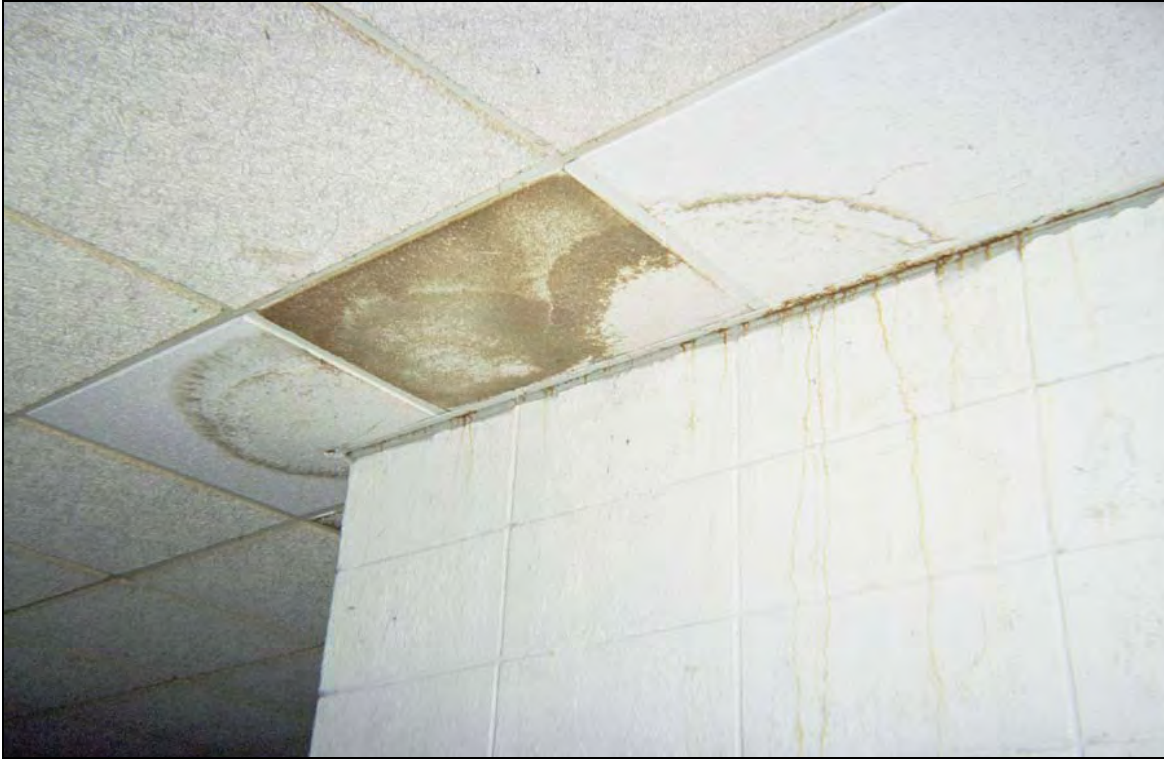
Figure 18: Interior Bathhouse - Ceiling Tiles
