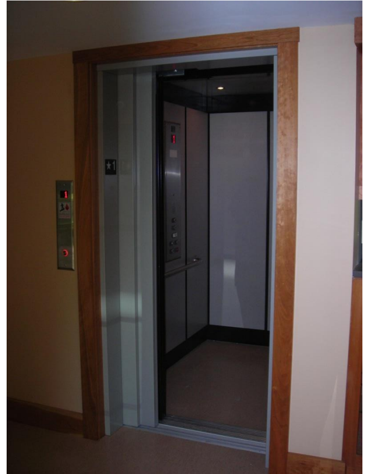
The elevator in the addition provides wheel chair access to several second floor historic rooms
