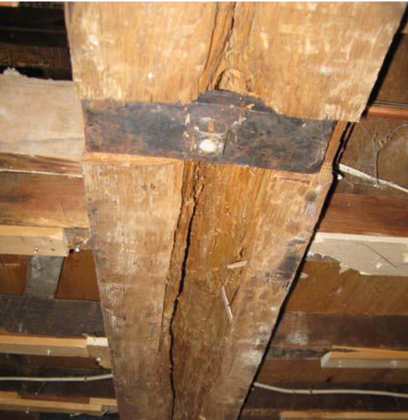
Rotted kitchen beam with tie rod to attic
