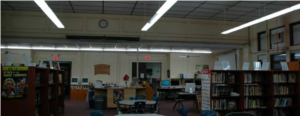
Figure 5: The rear wall and balcony of the original auditorium in the existing library space. The original ceiling is still in place above the dropped acoustic tile.
