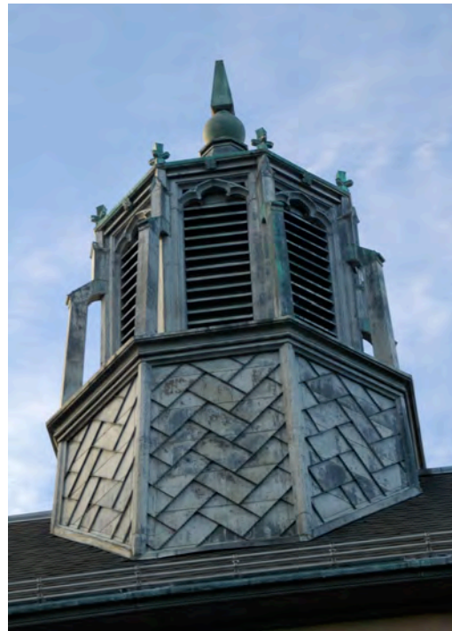
Figure 4: Close-up view of cupola.
