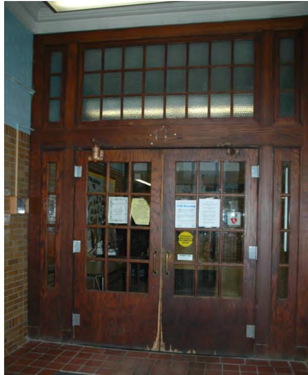
Figure 3: like many of Newton's school buildings of this era, the stairs are separated from the corridors with double doors, sidelights and transom panels.
