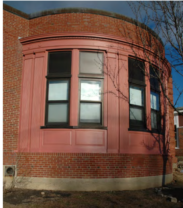
Figure 2: the bowed, single-story front projection with wood detailing is distinctive to this school
